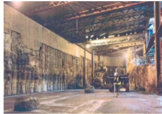
Sub-basement blinded, piles to be trimmed for stanchions to support first basement perimeter bays yet to be built.
