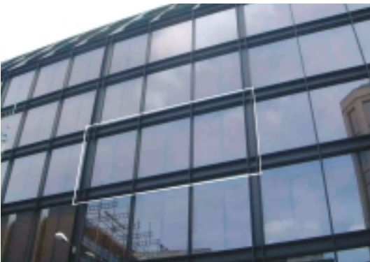
10 Gresham Street 9 m wide 4 m high finished cladding delivered from Germany. Rigid units bearing on slab adjacent the stanchions.
