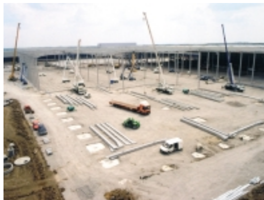
Erection taking place on four work fronts, with steel lay down areas for each gang
