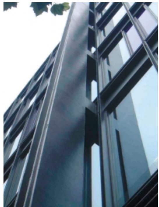
Mid City Place, Holborn with fabricated external box columns with rigid box beam spigots through the cladding spliced internally to floor beam.
