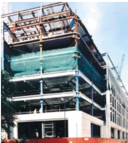
Deck bundles delivered to 6th; 5th floor decked; 3rd concreted. Cladding to 3rd floor.
