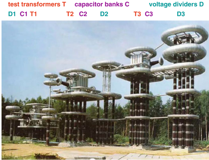
Fig. 3.15 World’s largest transformer cascade for 3,000 kV/4.2 A with capacitor banks for SI voltage generation
