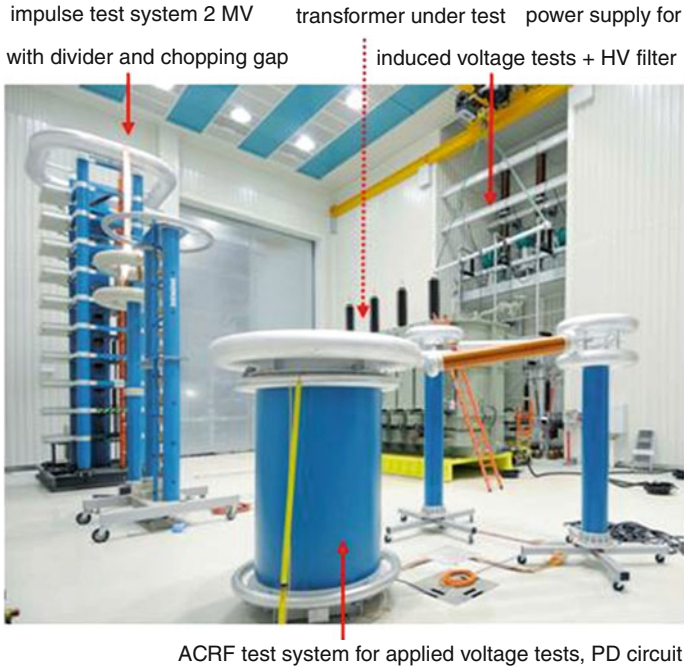
Fig. 9.9 Test field for routine and type tests on power transformers (courtesy Siemens AG, TBD Dresden)
