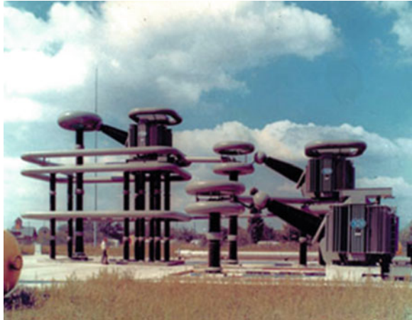
Fig. 9.30 Outdoor transformer cascade 1,800 kV/1.25 A (courtesy of Siemens AG, Berlin)
