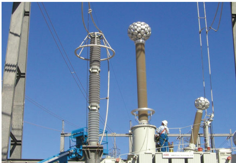
Fig. 4.36 Shielding electrodes assembled at the top of the bushings of a 500 kV single-phase transformer to avoid corona discharges disturbing the PD test
