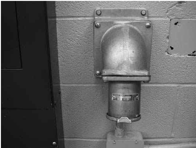
Figure 1-10 High-voltage, three-phase electrical outlet.
