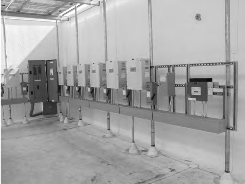
Figure 5.11 Water and Life Museum, distributed inverter systems. Photo courtesy of Vector Delta Design Group, Inc.
