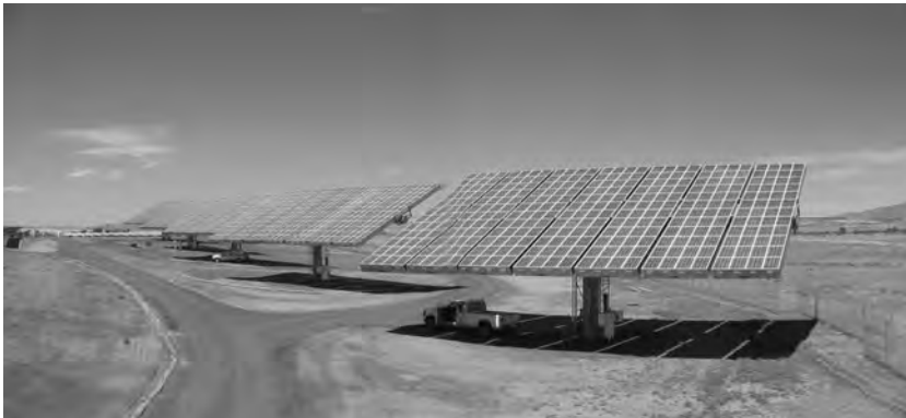
Figure B.22 30 KW Solar mega concentrator power co-generation farm. Photo courtesy of AMONIX.
