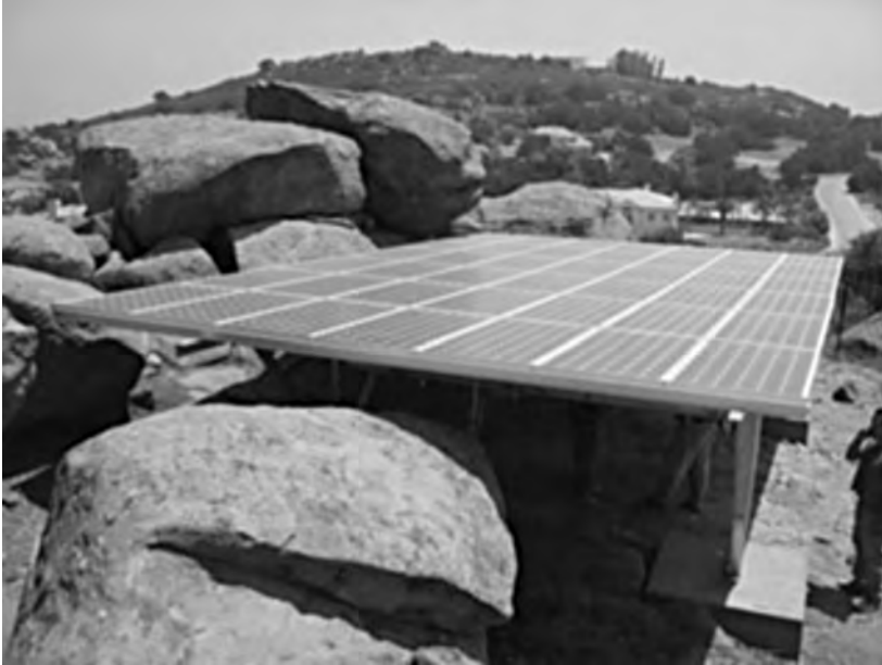
Figure B.23 Solar power system installation blended in rock bolder. Photo courtesy of California Green.
