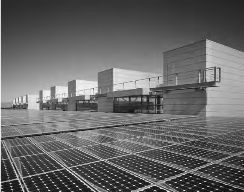
Figure 7.9 Water and Life Museum roof-mount solar power system. Engineered by Vector Delta Design Group Inc. Photo courtesy of Fotoworks.
