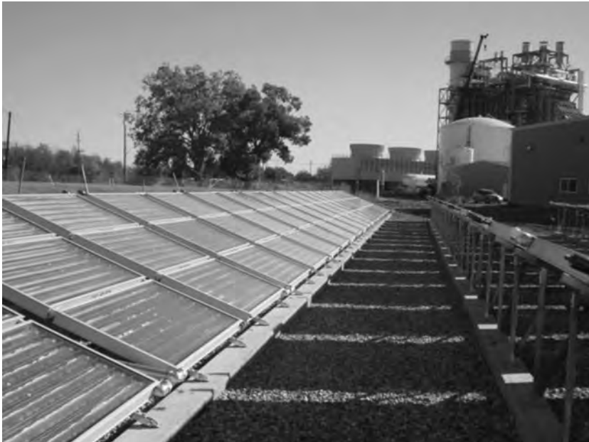
Figure 10.8 An industrial solar liquid heating panel installation.
