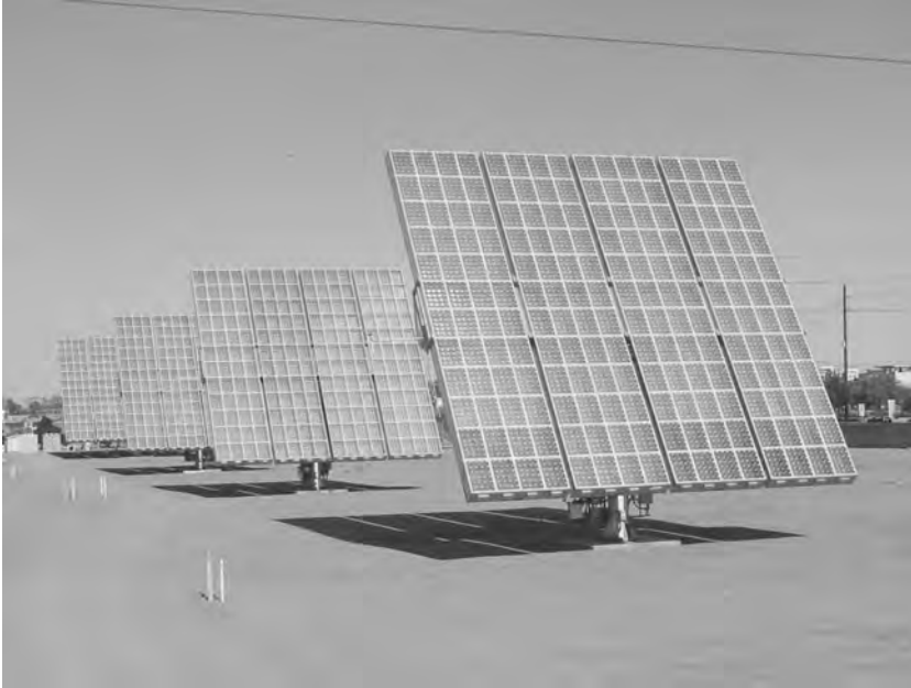
Figure 2.11 Amonix MegaConcentrator solar farm. Photo courtesy of Amonix.
