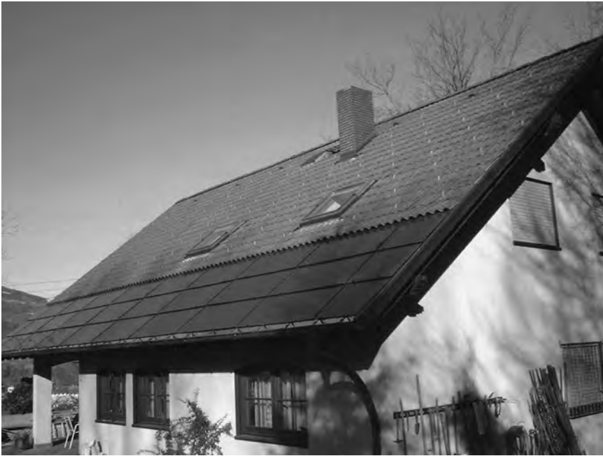
Figure 2.21 Roof-integrated MegaSlate photovoltaic system. Photo courtesy of Atlantis Energy Systems.
