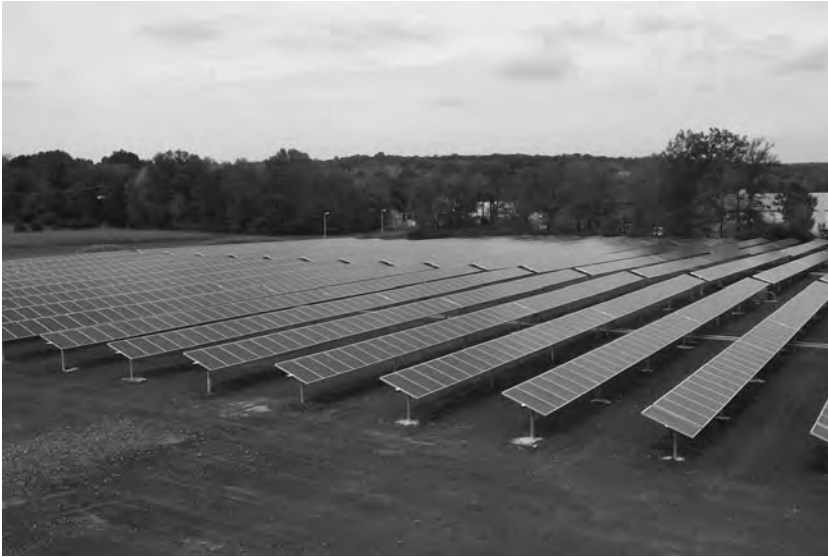
Figure B.34 Ground-mount single axis tracker solar power system.
