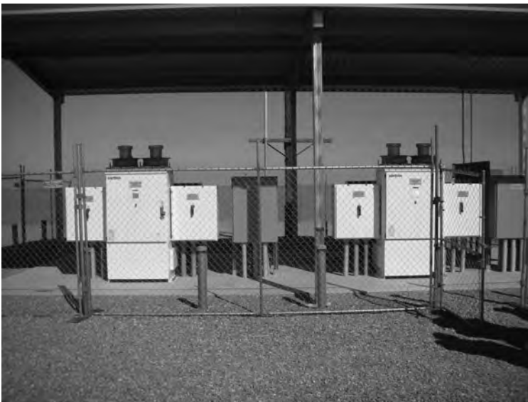
Figure 5.21 Solar power inverter installation, Semitropic Water District, Wasco, California. Photo courtesy of Vector Delta Design Group.
