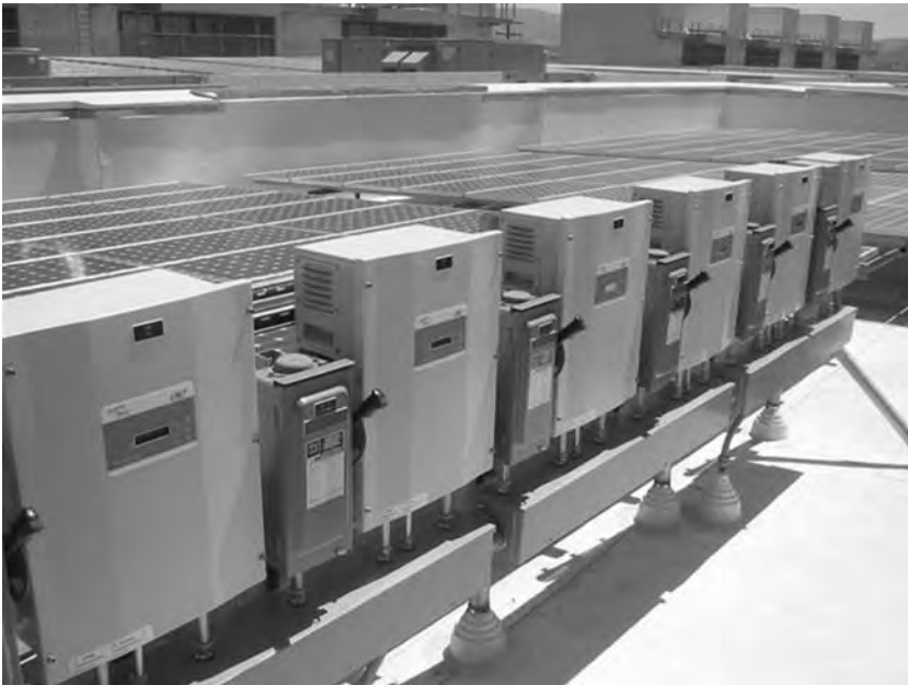
Figure 5.10 Water and Life Museum, rooftop solar power module and inverter installation. Photo courtesy of Vector Delta Design Group, Inc.
