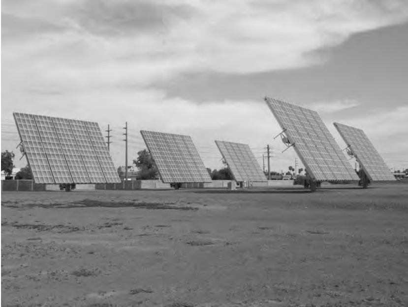
Figure B.21 25 KW Solar mega concentrator power co-generation farm. Photo courtesy of AMONIX.
