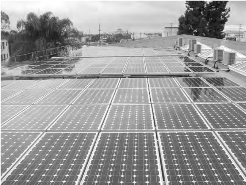
Figure 5.5 Roof-mount solar power system, Arshag Dickranian School, Hollywood, California. Photo courtesy of Vector Delta Design Group, Inc.
