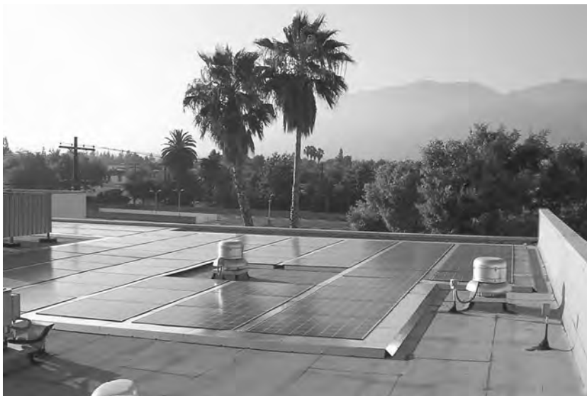
Figure 7.4 TriCom roof-mounted solar power cogeneration system.
