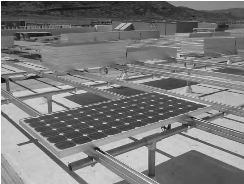
Figure 1.7 Photovoltaic panel module assembly mounted on a galvanized Unistrut channel.
