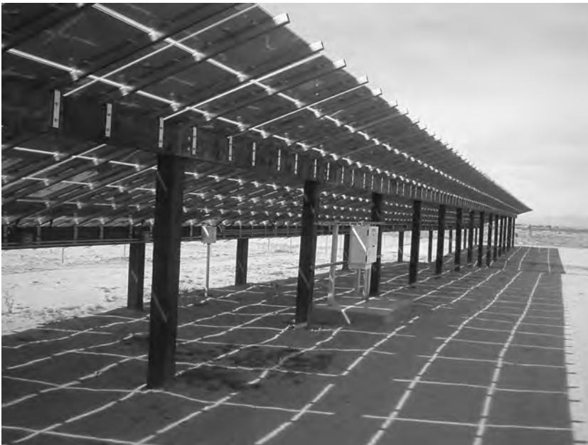
Figure B.24 Solar power farm installation in Mojave Desert. Photo courtesy of Grant Electric.
