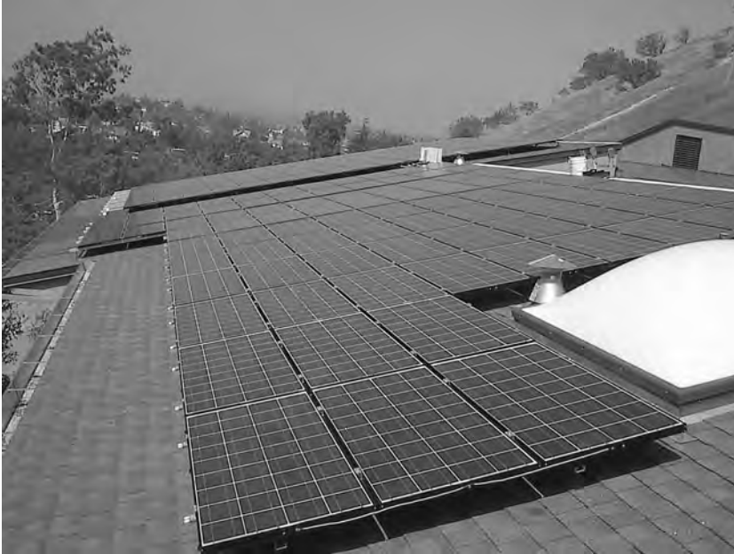
Figure 7.2 Los Angeles Audubon Center grid-independent solar power generation, system. Photograph courtesy of LA Audubon Society.
