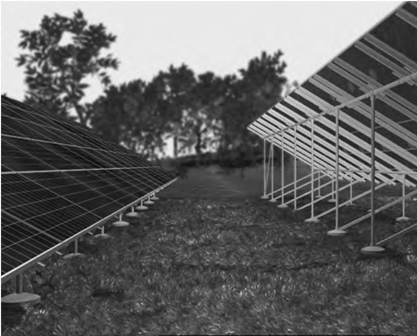
Figure 9.7 Typical solar power farm installation. Graphics courtesy of UNIRAC.
