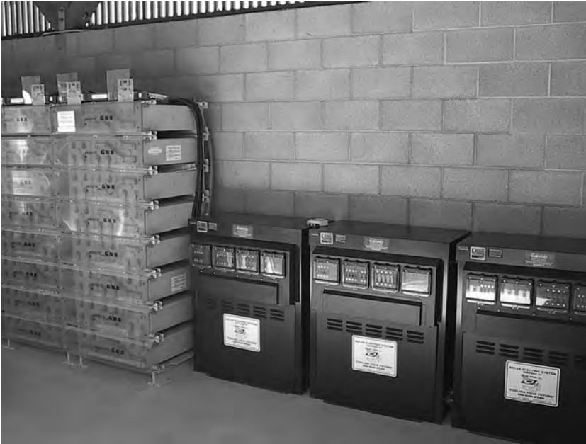
Figure 3.11 Deep-cycle battery bank system. Courtesy of Solar Integrated Technologies.
