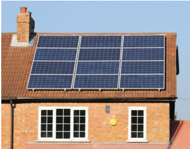
Figure 11.14 Monocrystalline PV array.
