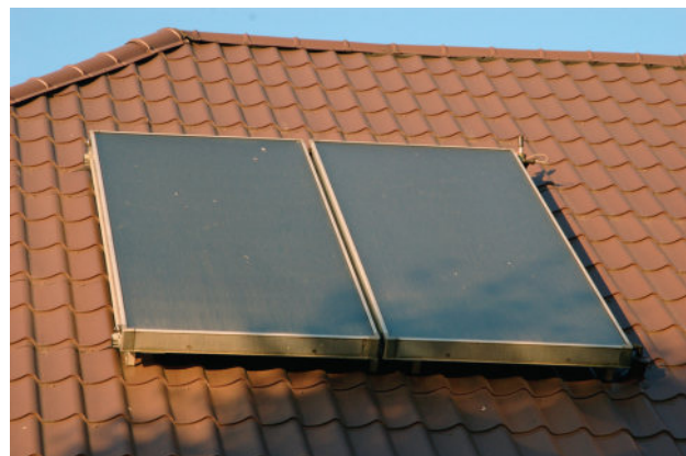
Figure 11.10 Flat plate solar thermal panels.
