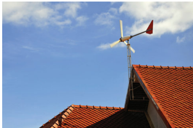
Figure 11.17 Mast mounted turbine.
