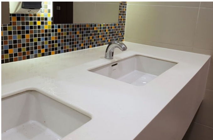
Fig. 8.2 Photo showing a sensor controlled water tap
