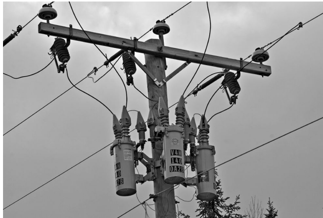
FIGURE 5-2 Three-phase transformer array.
