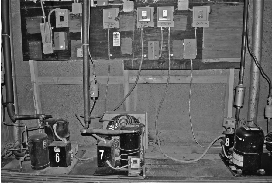
FIGURE 13-3 Three air-cooled compressors in a compressor room.
