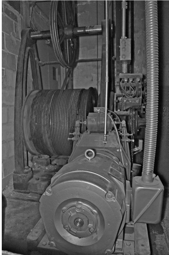
FIGURE 11-1 Elevator motor with cable drum.
