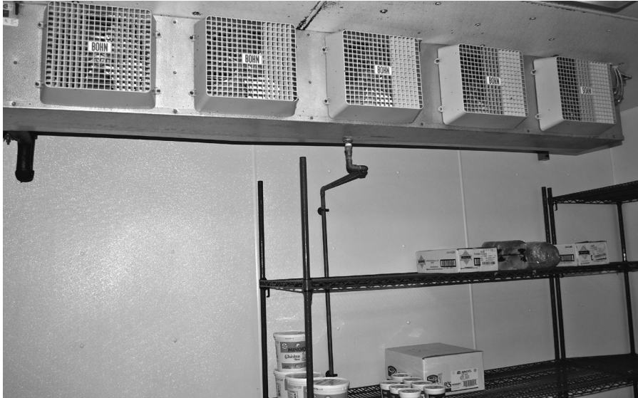
FIGURE 13-2 Five evaporators in a walk-in cooler.
