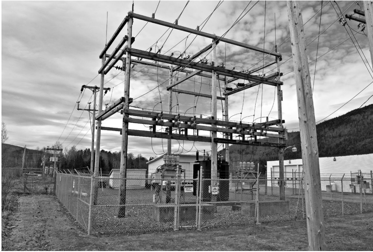
FIGURE 5-1 Substation with grounded fence.
