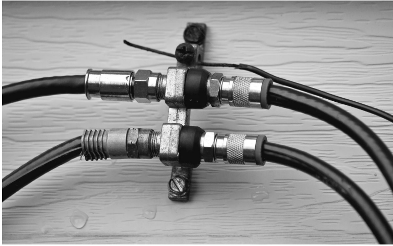
FIGURE 10-2 Satellite dish primary protector on an outside wall.
