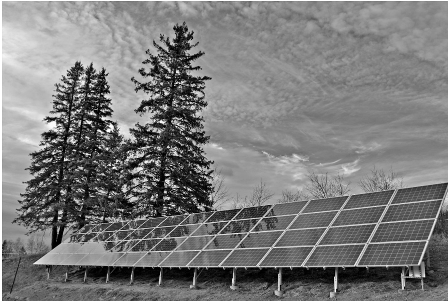
FIGURE 15-2 Solar PV array.
