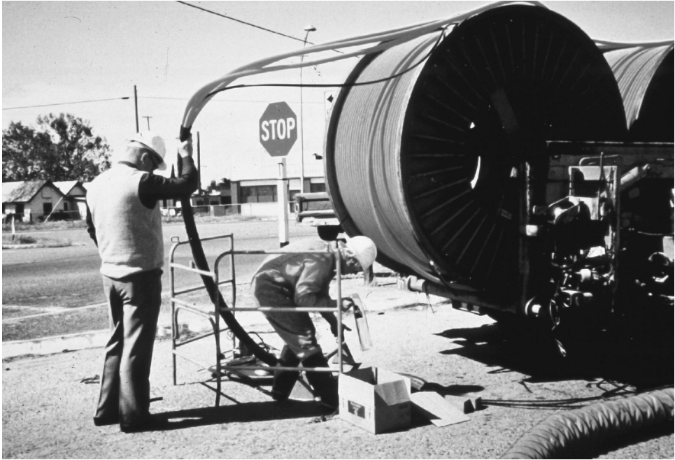
FIGURE 17-2 Long outside fiber optic runs require precision splices. (Courtesy of Fiber Optics Association.)
