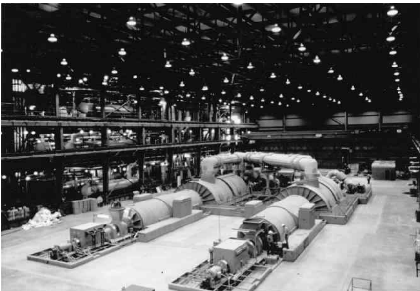
FIGURE 1.4 An installed 1300MW cross-compound turbine generator.
