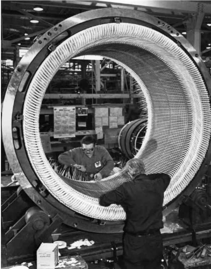
FIGURE 7.4 Winding the stator of a synchronous generator. (Courtesy of MagneTex, Nashville, TN.)
