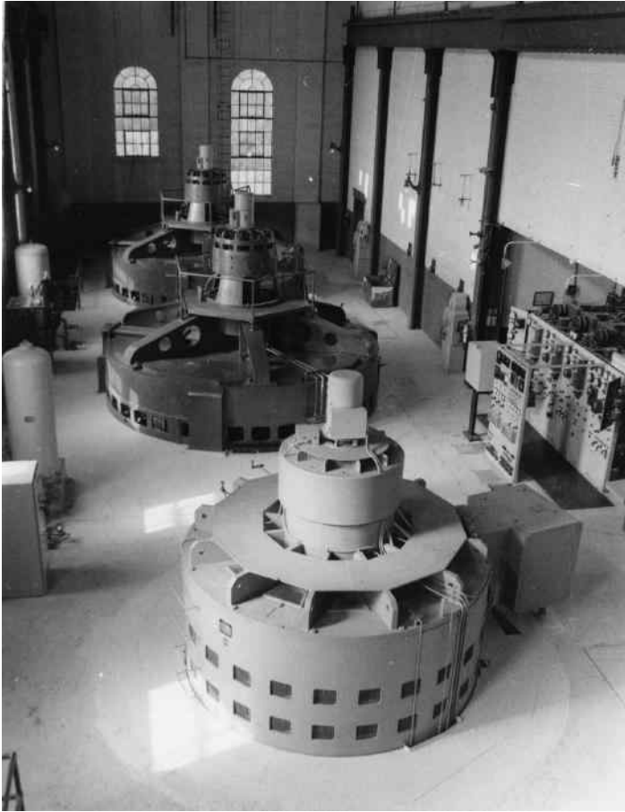
FIGURE 5.8 A vertical synchronous generator used by a large industrial firm. (Courtesy of General Electric Canada, Inc., Mississauga, Canada.)
