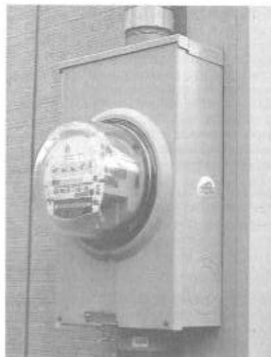
Fig. 8-7 Typical outdoor weatherproof kilowatt-hour meter and its socket.
