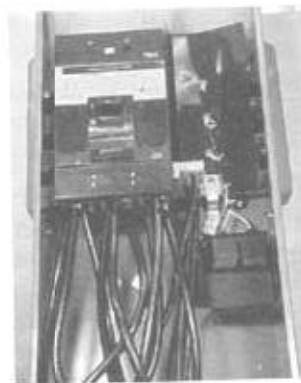
Fig. 17-8 A surge (lightning) arrester installed in a service switch cabinet. Be sure its white wire is connected to the grounded neutral busbar in the cabinet. Take care to terminate its wiring at appropriate terminals; most main circuit breaker lugs are not listed for the combination of the small wires from the arrester and the much larger feeder or service conductors. Consult with the panelboard manufacturer for availability of appropriate terminations for the surge arrester. (Square D)
