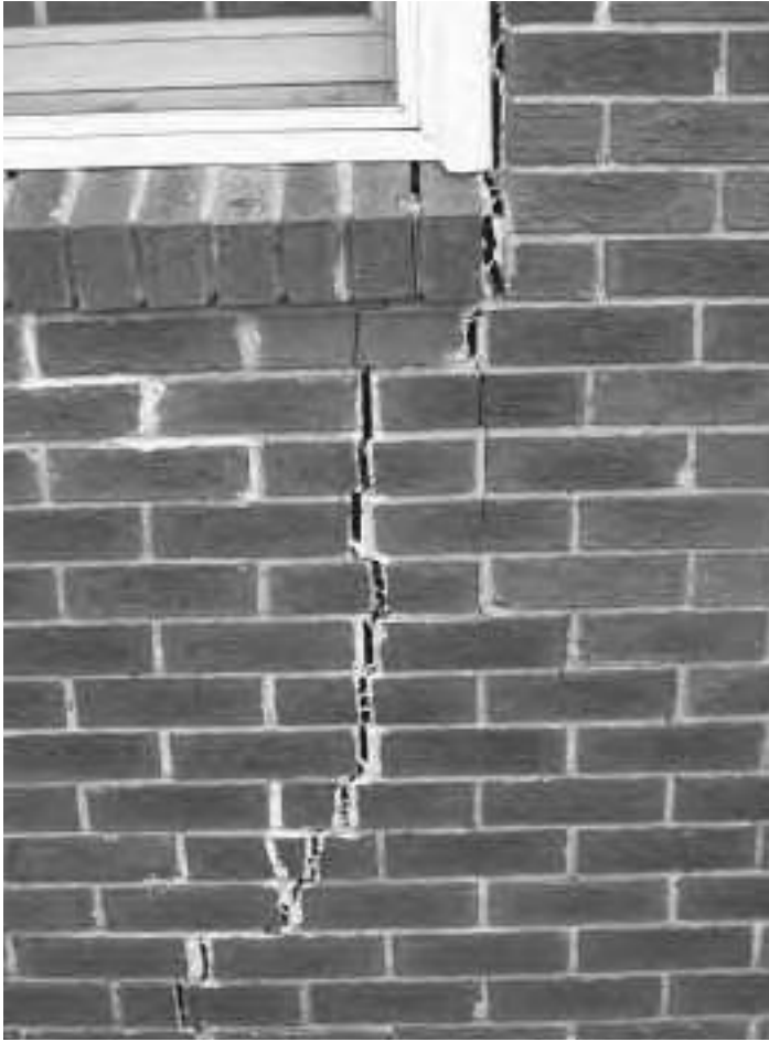
Shrinkage of expansive clay soil resulted in soil movement and structural damage to this home.
