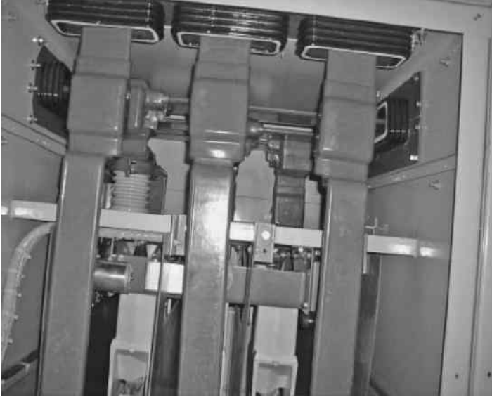
FIGURE 7.9 High-voltage bus bars in switchgear through porcelain bus ducts: cast epoxy insulated with joints covered by removable boots. (From Myers Power Products, Inc. With permission.)
