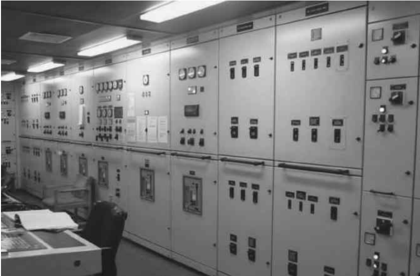
FIGURE 7.13 Typical main switchboard on large cargo ship. (From Raul Osigian, U.S. Merchant Marine Academy.)
