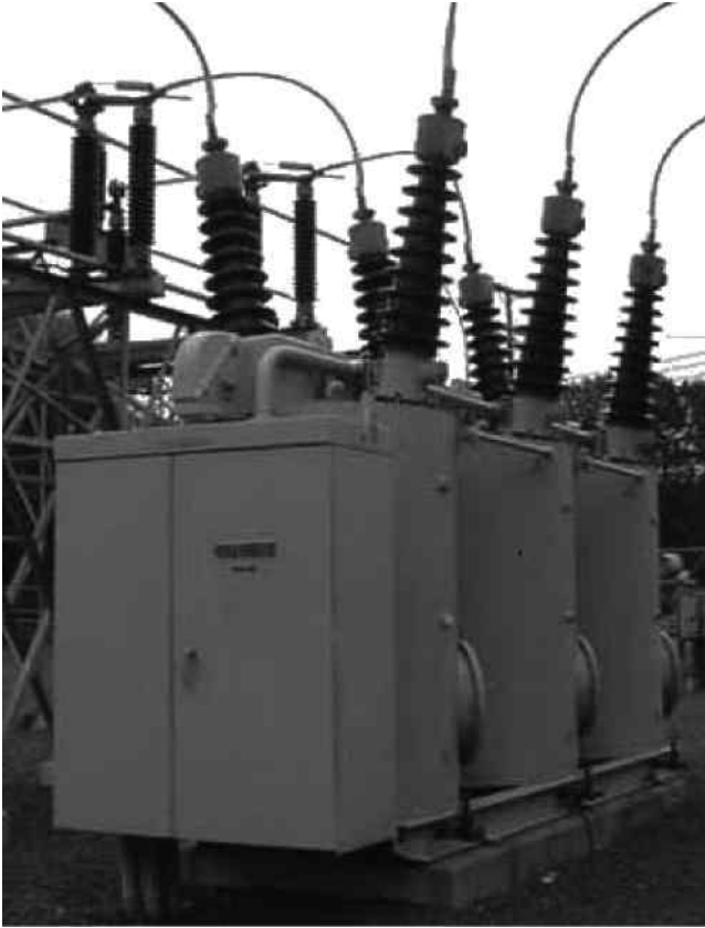
FIGURE 9.13 HV oil circuit breaker in outdoor substation yard.
