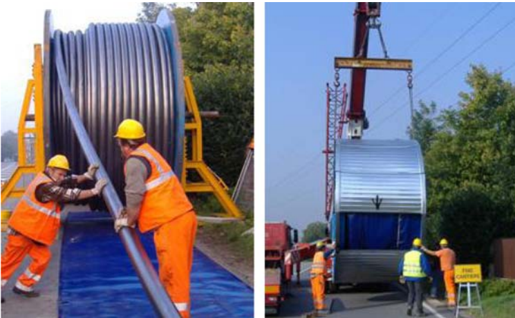
Figure 1.25 (Turbigo–Rho mixed line) Cable drum (Courtesy of TERNA)
