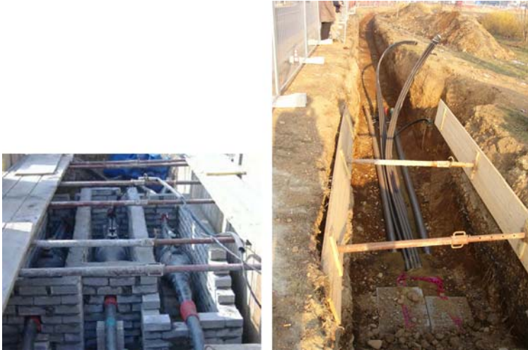
Figure 1.27 (Turbigo–Rho mixed line) Joint location and trench (concrete slabs are also visible) during installation phase (Courtesy of TERNA)
