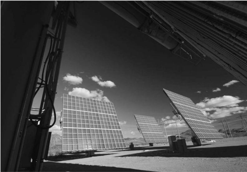
Figure 8.26. A dual axis solar power system.
