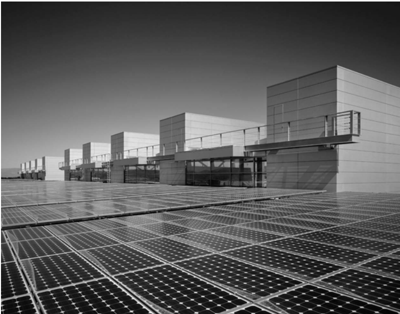
Figure 3.7. A roof mount solar power system. Source: Vector Delta Design Group, Inc.
