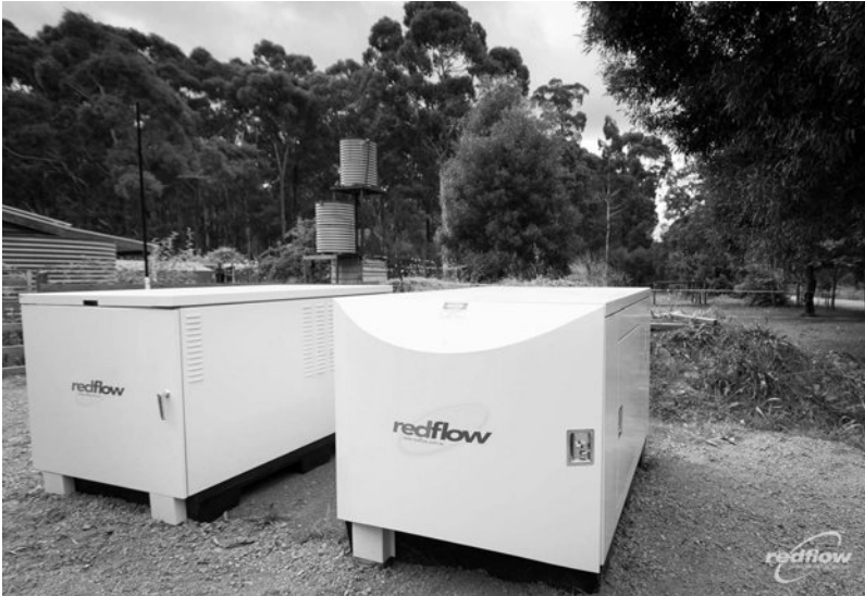
Figure 12.22. Zinc-bromine battery installation.
