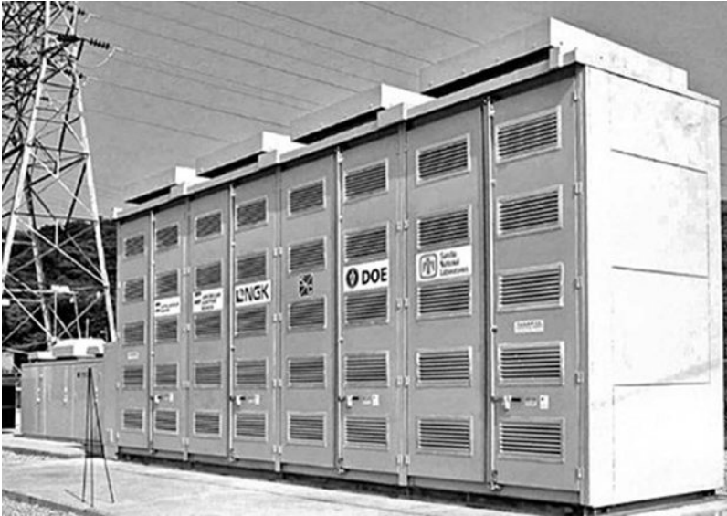
Figure 12.18. Sodium sulfur battery installation. Source: Courtesy of NGK Japan
