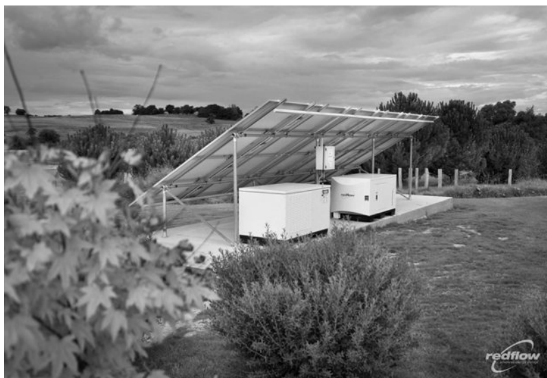
Figure 12.23. Zinc-bromine battery installation in solar power system application. Source: Photo courtesy of Redflow
