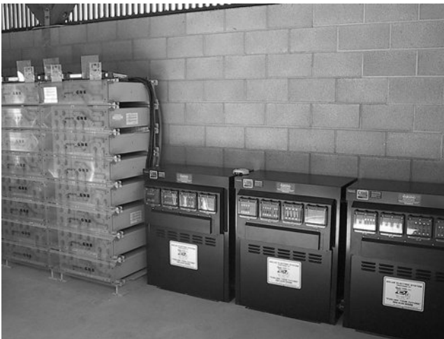
Figure 12.3. Deep-cycle lead acid battery pack.
