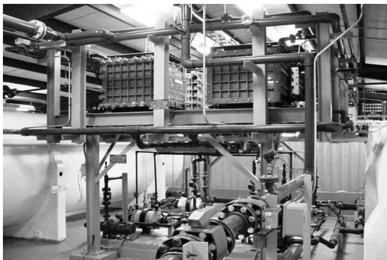
Figure 12.20. A 200-kW vanadium redox flow battery installation. Source: Photo courtesy of VRB-ESS, Utah, United States
