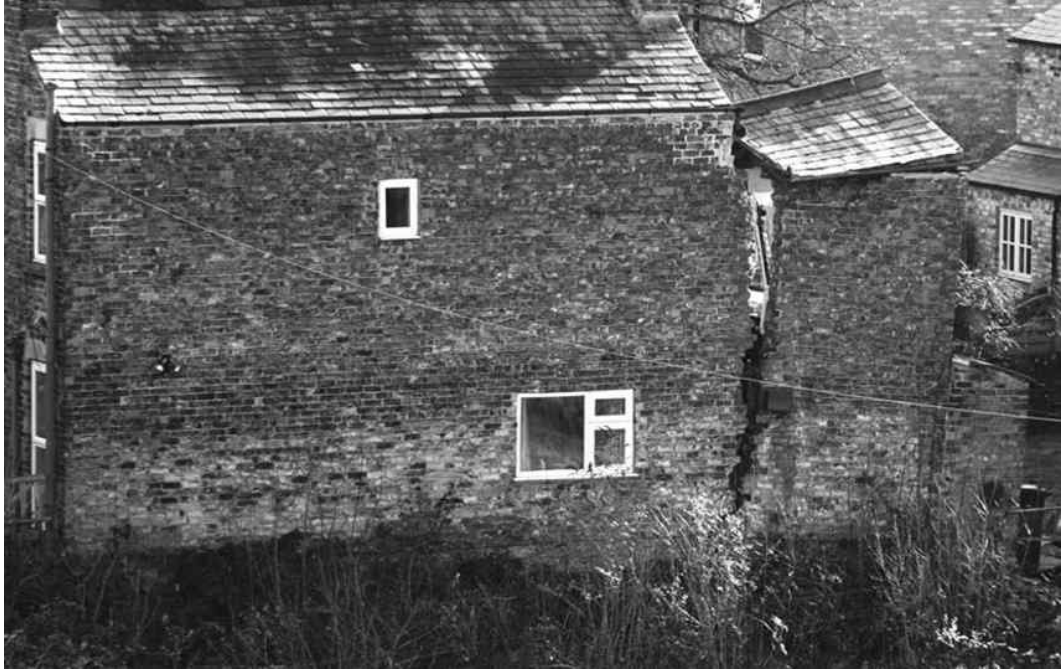
Figure 12.1: Photograph showing damage caused by a sinkhole in Ripon, Yorkshire. By kind permission of The Press, York.
