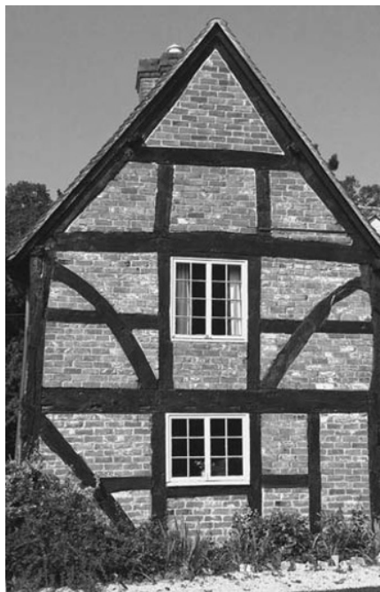
Figure 3.10: A property constructed circa 1600s with convex knee brace and queen post truss.
