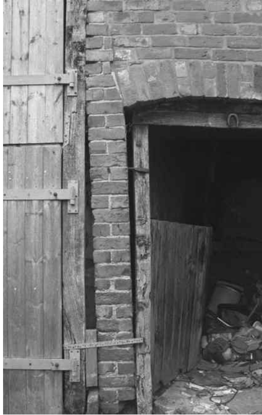
Figure 11.4: Photograph showing failure of abutment due to arch thrust.
