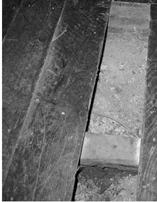
Figure 9.1: Photograph showing a timber floor laid directly onto earth in a Georgian property.
