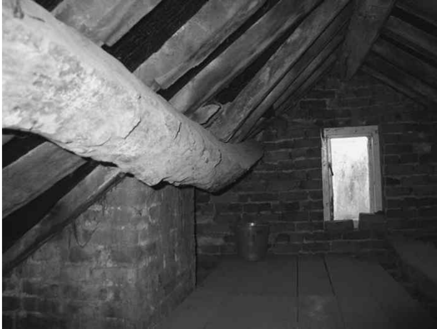
Figure 18.6: Photograph of a deflected purlin.
