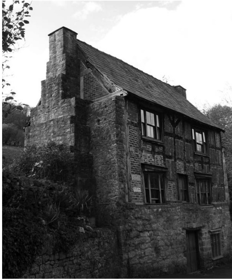
Figure 3.17: Photograph showing how a chimney offers lateral strength to a timber frame property.
