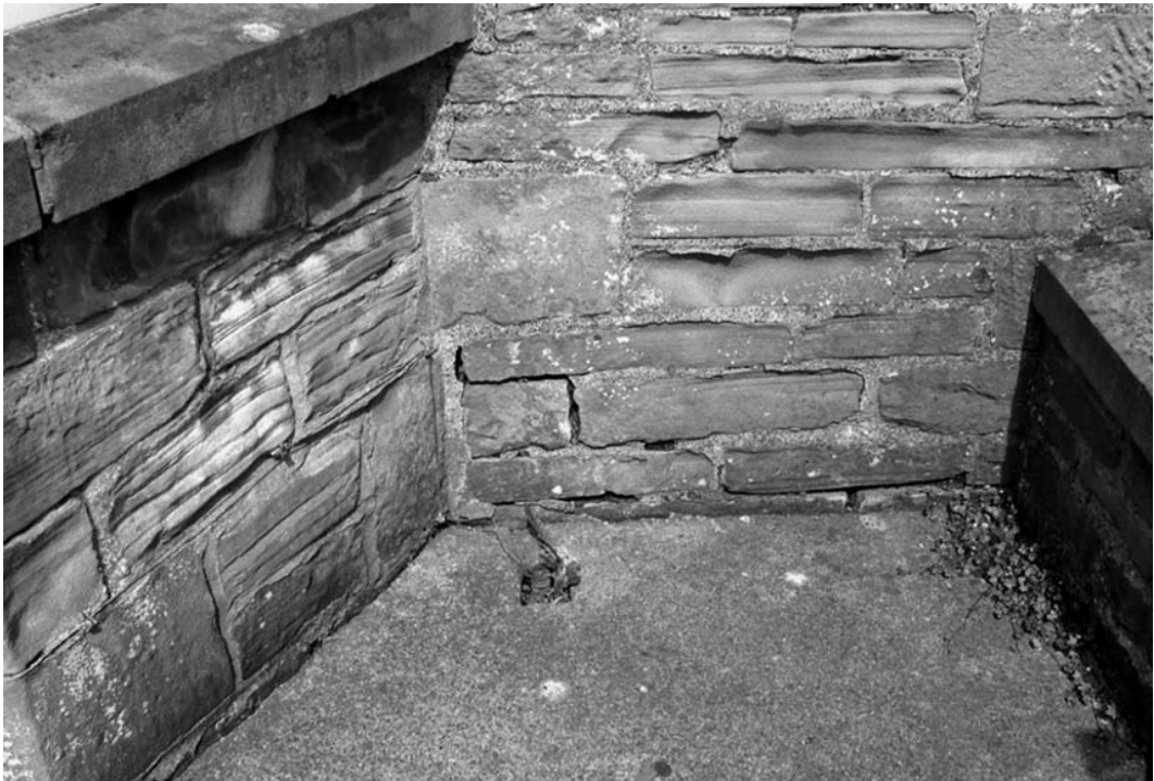
Figure 3.1: Damage caused by cement pointing.
