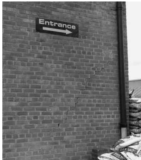
Figure 18.2: Photograph showing diagonal subsidence crack in a building.
