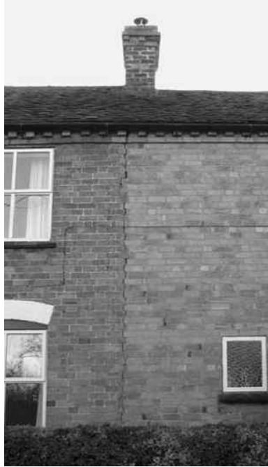
Figure 18.1: A tapered subsidence joint between the line of an extension.
