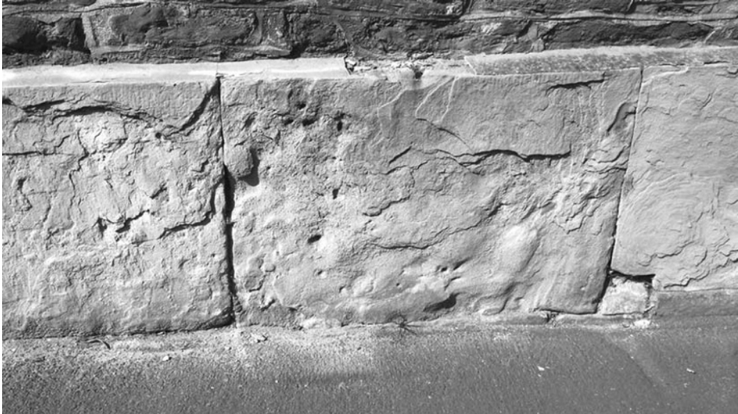
Figure 3.23: Photograph showing delamination of stone face due to vertical bedding.
