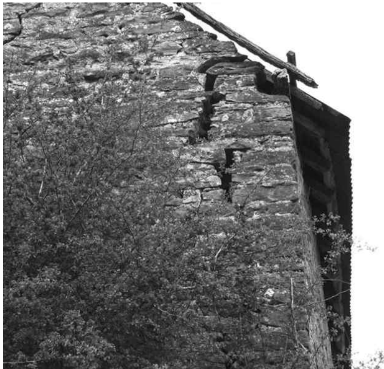
Figure 10.8: Photograph showing a property with roof spread.
