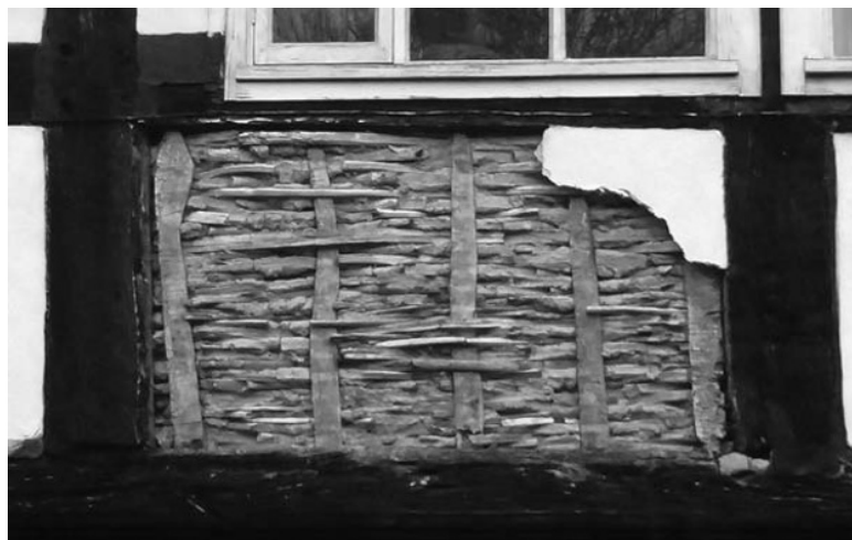
Figure 3.13: Photograph showing wattle and daub exposed on a damaged property in Herefordshire.
