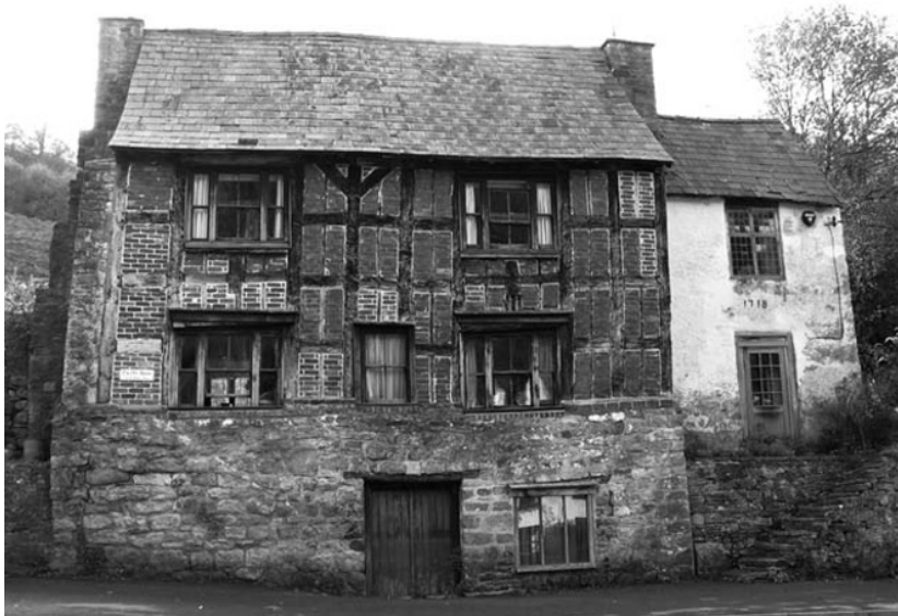
Figure 3.8: A timber frame building circa 1500s with an extension to the right-hand side dated 1718.
