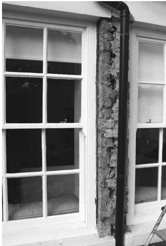
Figure 18.5: Photograph showing overloaded column of brickwork which has failed in compression.
