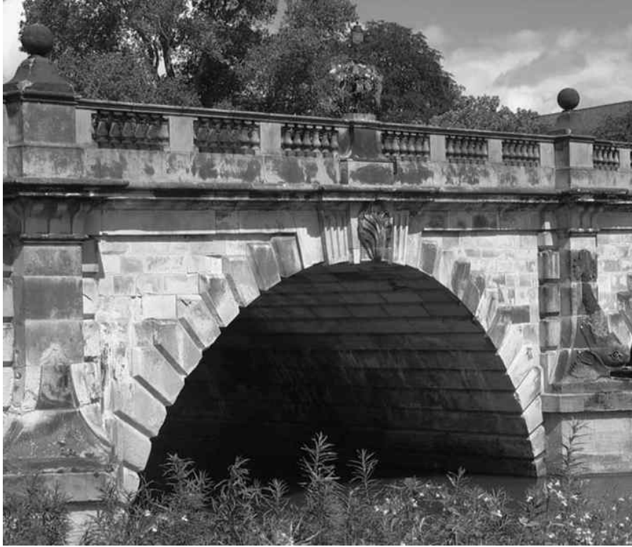
Figure 11.1: Photograph showing the keystones and voussoirs running through the length of the English Bridge at Shrewsbury in the formation of the arch.
