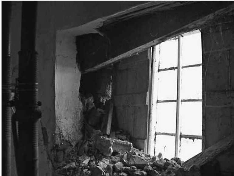
Figure 18.4: Photograph showing the loss of bearing of a beam subject to wet-rot deterioration.
