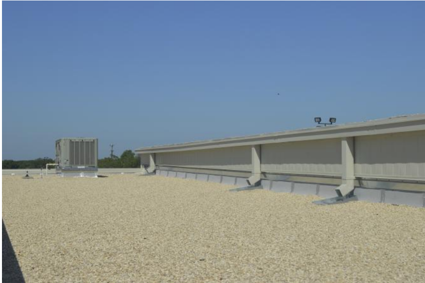
Figure 4.9 Typical design of a multilevel gravel roof. Over time, debris will accumulate on this roof. The degree to which this type of roofing material will affect water quality in the tank is determined by intensity of local rainfall and how well the roof is maintained. (Eddie Van Giesen)
