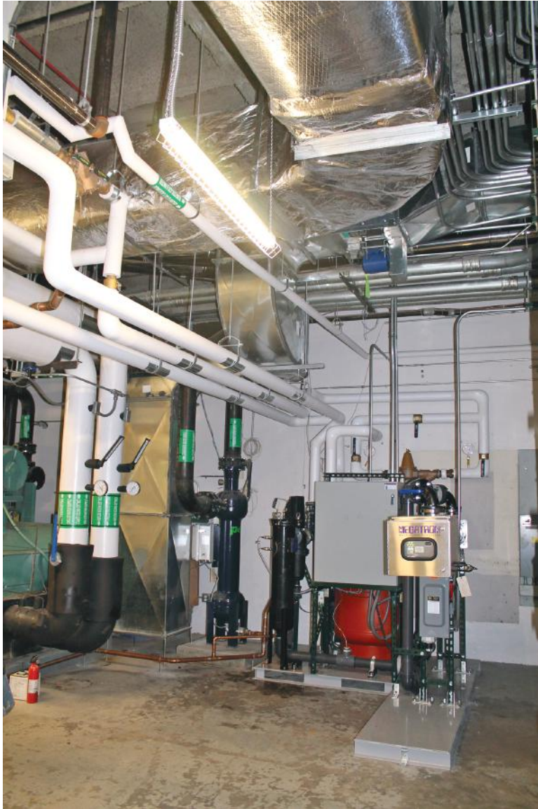
Figure C.12 Rainwater harvesting equipment area in mechanical room at the College of Environment and Design at the University of Georgia, Athens. ( Celeste Allen Novak )
