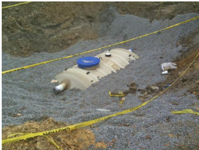
Figure 4.26 Care must be taken during construction to prevent introduction of mud and debris into tank. Note that this inlet pipe is temporarily covered during construction. (Eddie Van Giesen)
