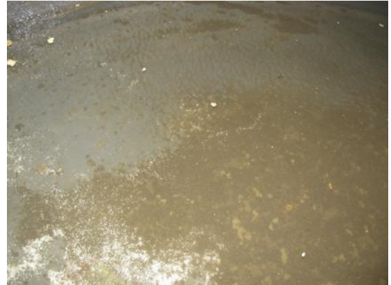
Figure 5.6 Sediments and organic matter accumulate on the bottom of rainwater storage tanks and can become a source of contamination. ( Kathy DeBusk )
