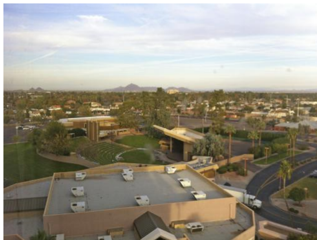
Figure 4.19 Typical commercial roof with HVAC commercial rooftop units. Contaminant loads exiting commercial roofs are highly variable, depending on locale and rooftop inspection and maintenance. (Eddie Van Giesen)
