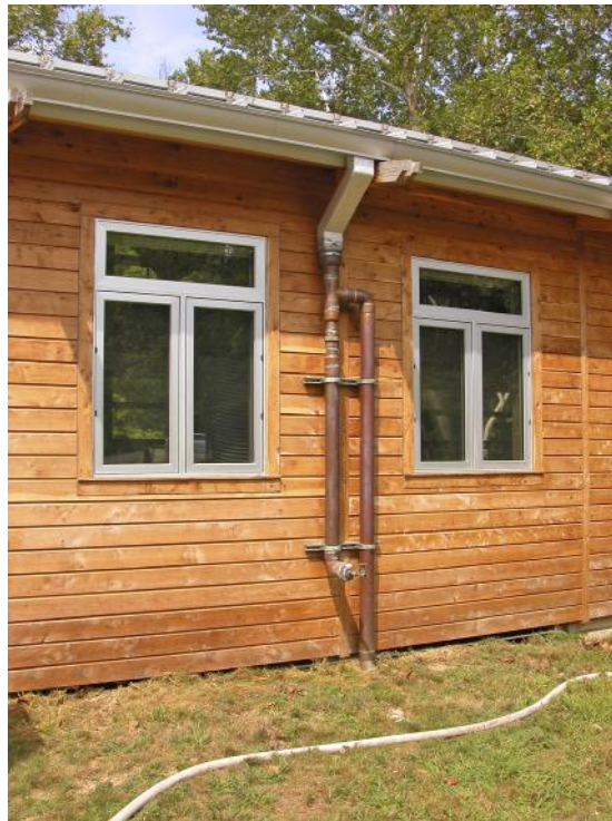
Figure 5.19 Tyson Living Learning Center downspouts with rain diverter. (Ralph Bicknese, Hellmuth + Bicknese Architects)
