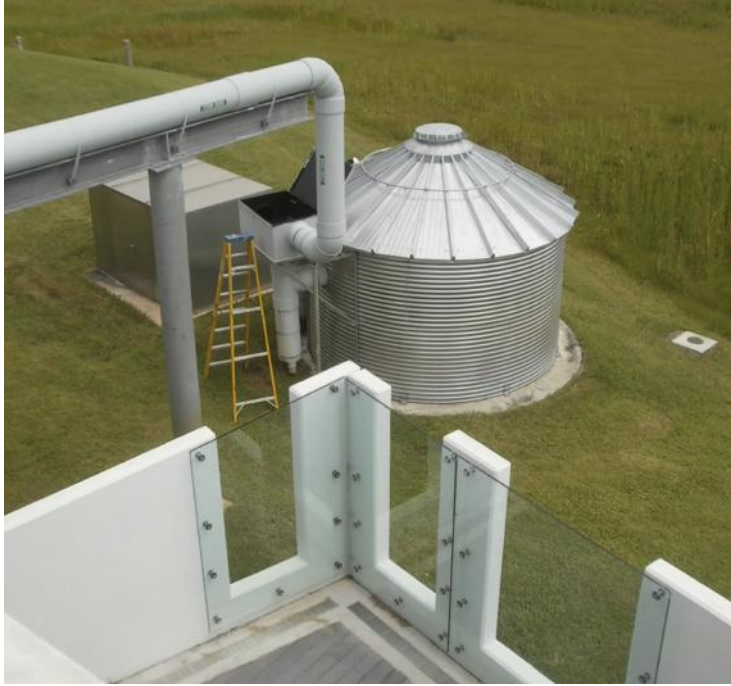
Figure 4.10 Water is conveyed from a butterfly roof to storage at the Young At Art Museum. (Eddie Van Giesen)
