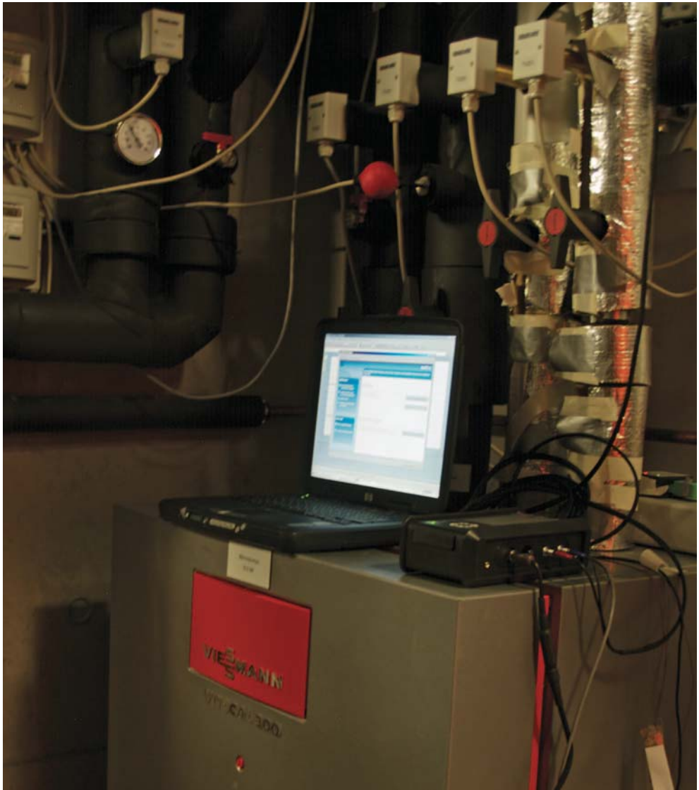
Figure 8.2 Heat pump with vertical ground heat exchangers in the youth centre Ostfildern (Photo: Barta).
