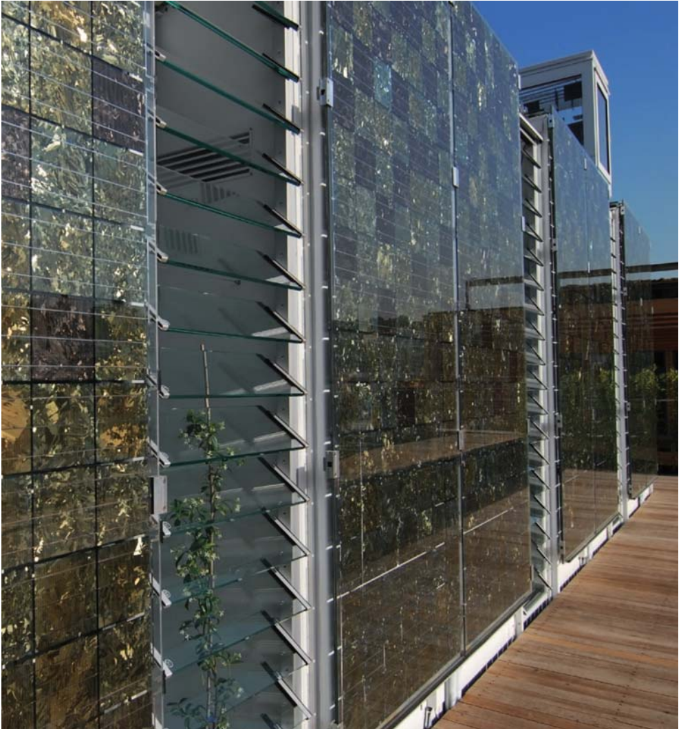
Figure 7.2 PVT facade of the experimental SDE House on location in Madrid (photo: Jan Cremers, HFT Stuttgart), see also 9.6 Photovoltaic thermal collectors for heating and cooling generation on page 576.
