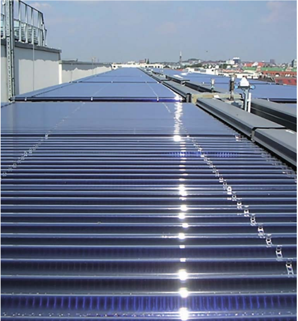
Figure 5.2 Vacuum tube collectors on the Presseamt in Berlin, Germany (Photo: Eicker).
