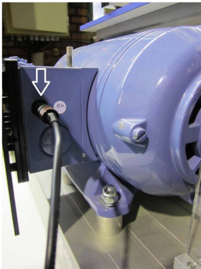
Figure 11. Temperature monitoring of a motor stator winding
