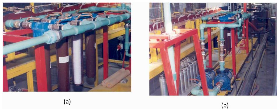
Figure 73. Cooling water filters
