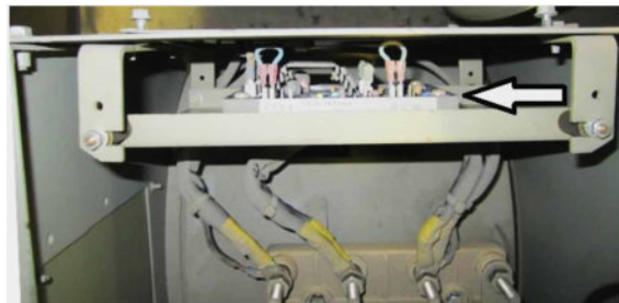
Figure 61. Mounting of a static rectifier used for rotor of a synchronous generator
