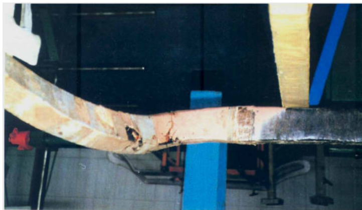
Figure 74. A damaged stator bar of a plant turbogenerator due to flashover
