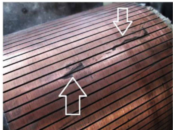
Figure 113. A damaged commutator of a DC generator
