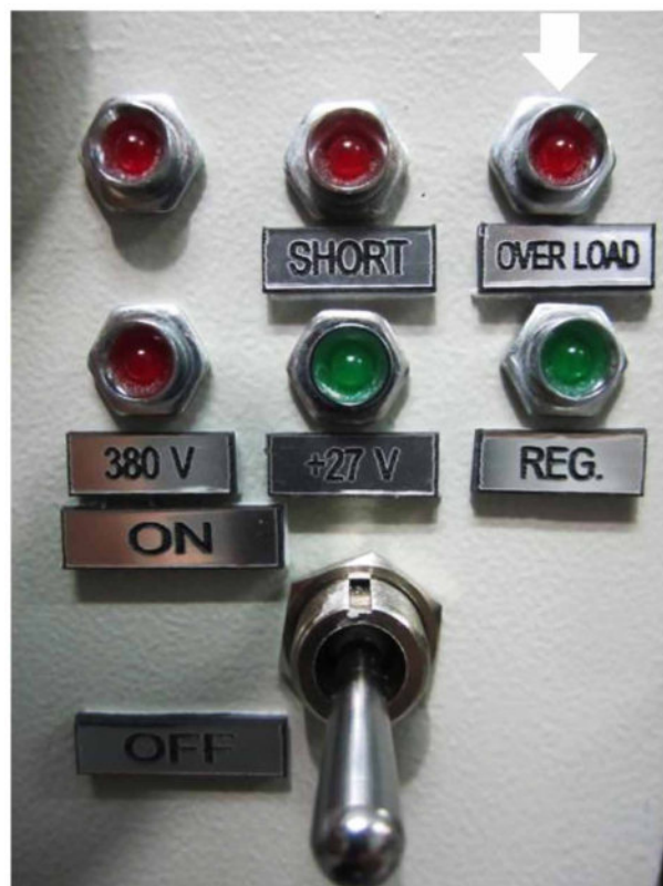
Figure 38. An operator panel with two levels alarms
