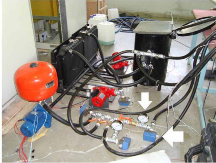
Figure 31. Water flow switches in a cooling system
