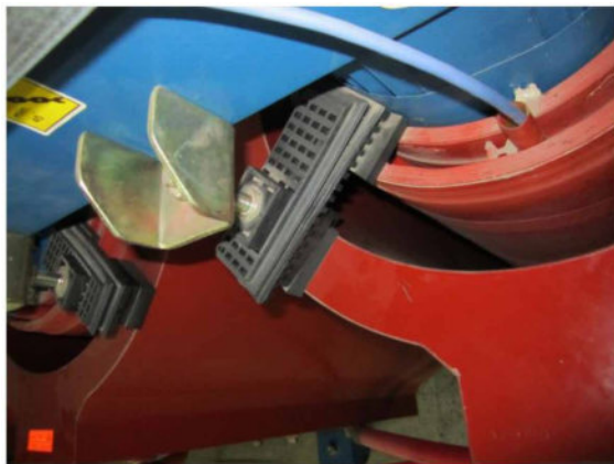
Figure 35. Cooling ducts in a three phase transformer
