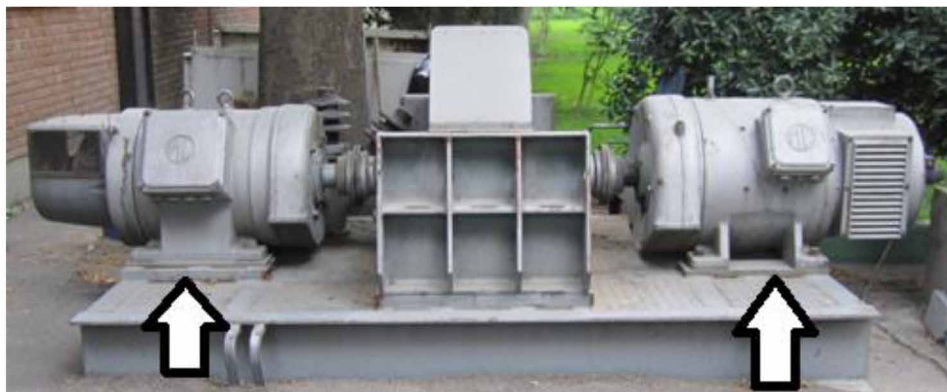
Figure 85. A rotary power converter used a UPS: DC motor supplied with batteries (right), three phase AC generator used as AC power supply (left)
