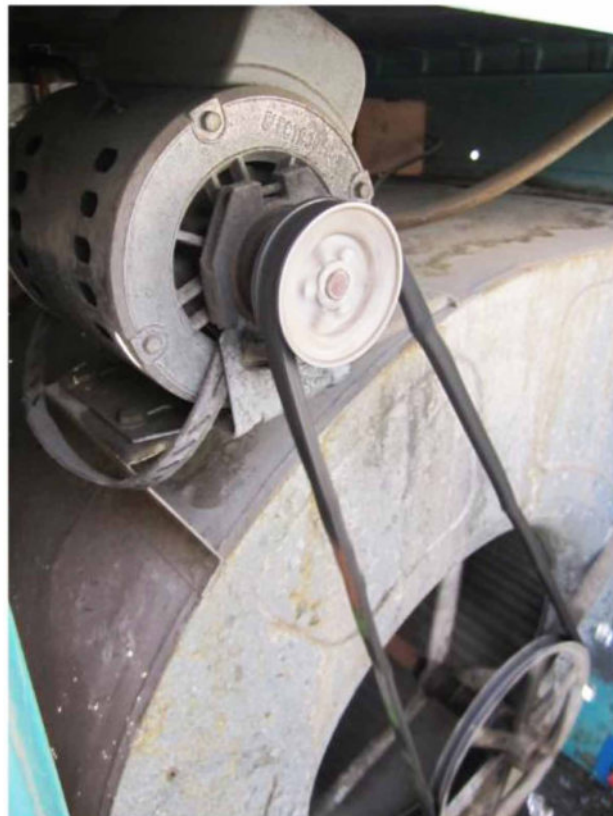
Figure 99. A cooling fan under stress
