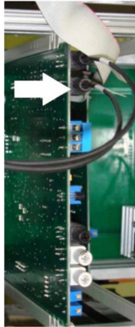
Figure 29. Application of fiber optic for isolated condition monitoring
