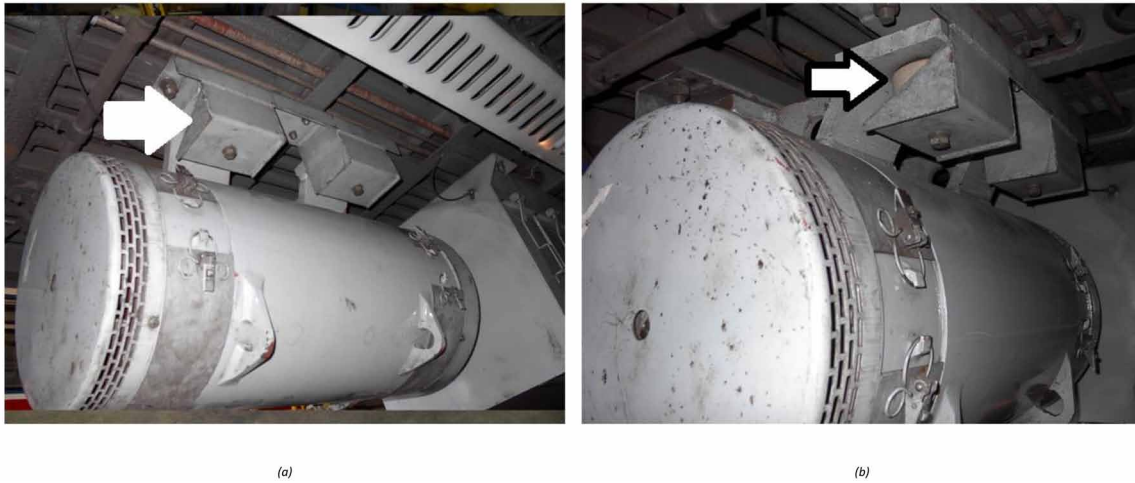
Figure 72. Application of damper for a rotary power supply in railway
