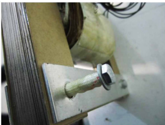
Figure 27. Isolation of laminated sheets in the core of a transformer
