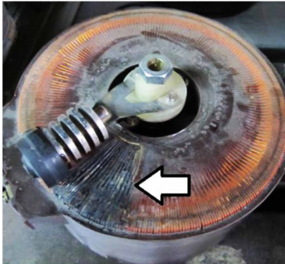
Figure 85. A damaged autotransformer due to humidity
