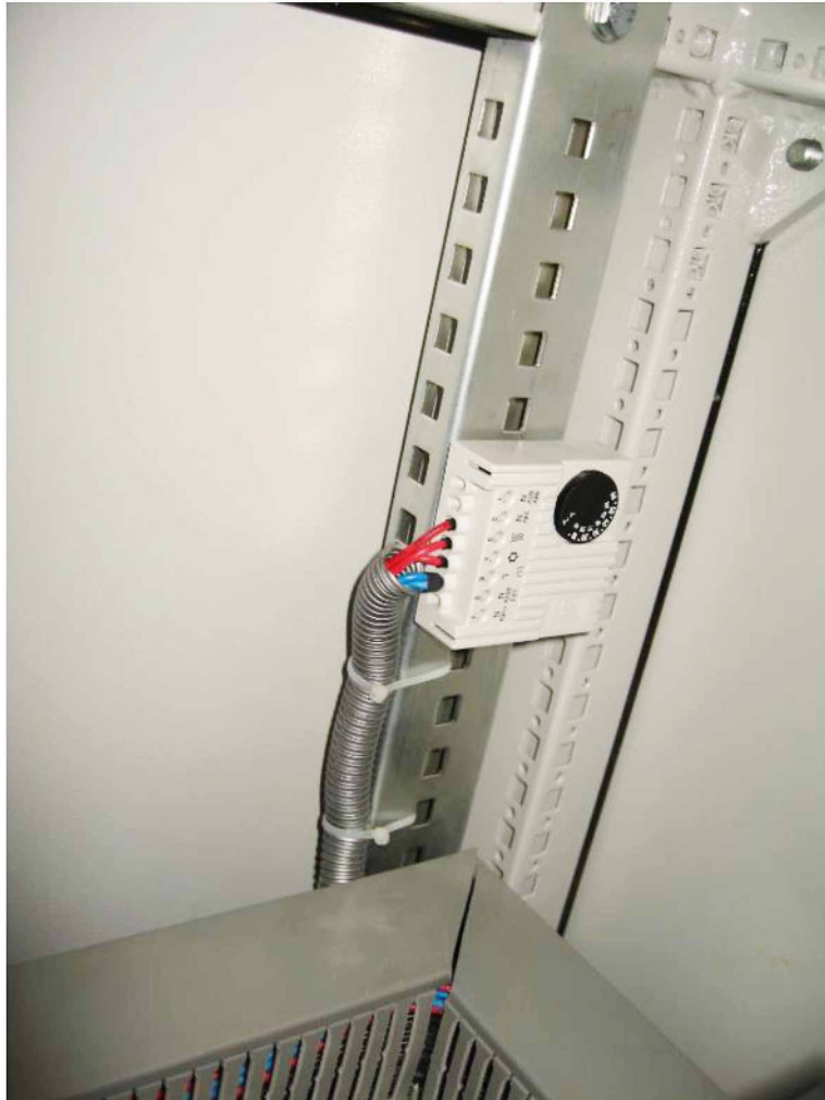
Figure 32. A temperature-humidity control used in a cabinet with communication application
