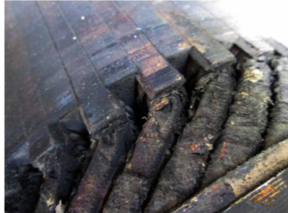
Figure 92. Effect of dust on rotor of a DC generator
