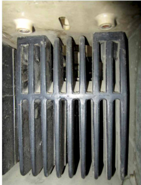
Figure 21. One of the heat sinks without galvanic isolation with high voltage switch in a rectifier with non-isolated heatsinks
