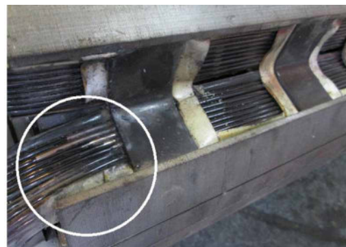
Figure 57. A damaged rotor winding due to electrical breakdown
