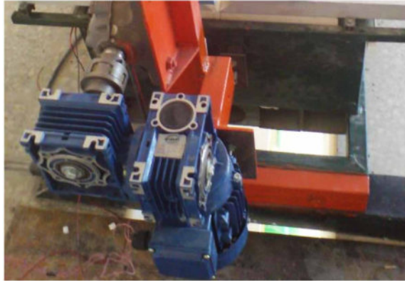
Figure 45. A very low speed motor affected by voltage harmonics
