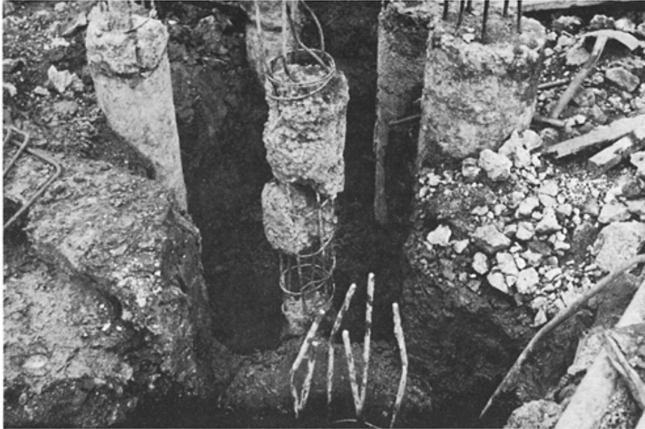
Fig. 3.39 Defective shaft of bored pile caused by cement being washed out of unset concrete
