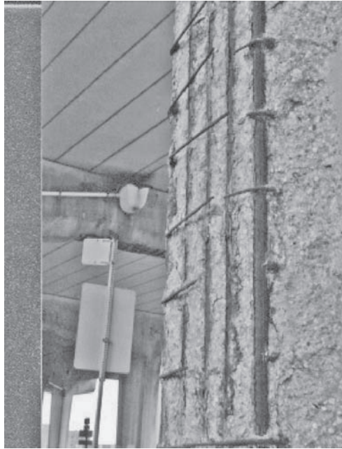
FIGURE 3.6 Photo of corrosion in concrete.
