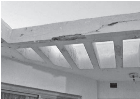
FIGURE 2.1 Deterioration in a reinforced concrete beam.
