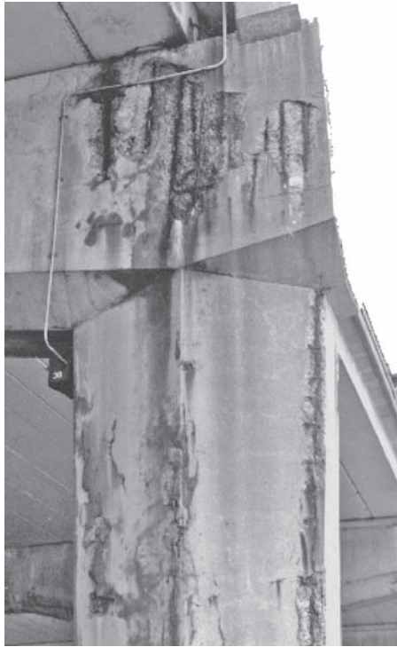
FIGURE 4.3 Brown spots on bridge column and girder.
