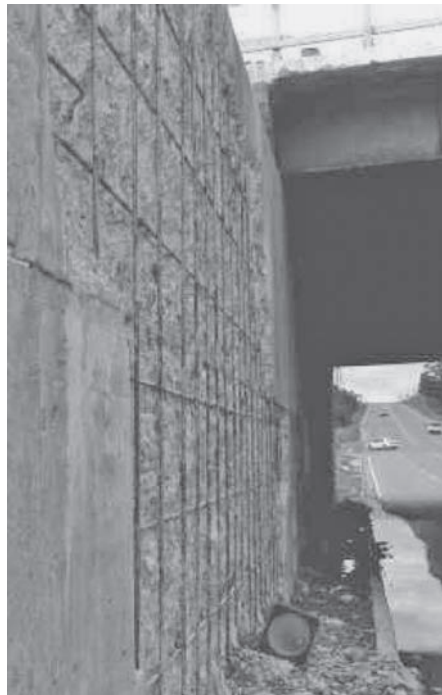
FIGURE 3.7 Photo of corroded abutment bridge wall.
