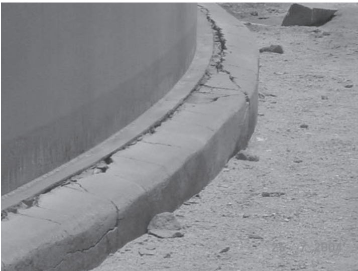
FIGURE 4.19b Cracks on the tank ring beam.
