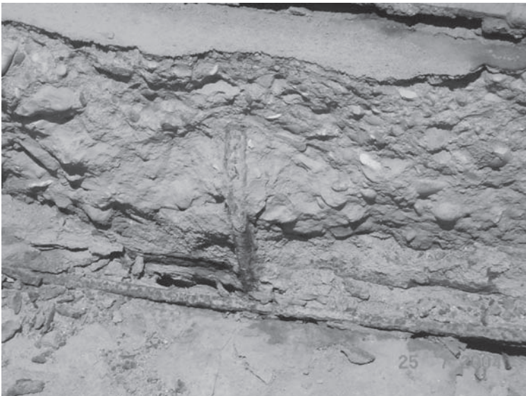
FIGURE 4.19d Reduction in steel cross-sectional area.
