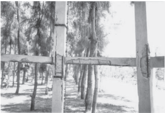
FIGURE 3.9 Photo of cracks on columns and beams.
