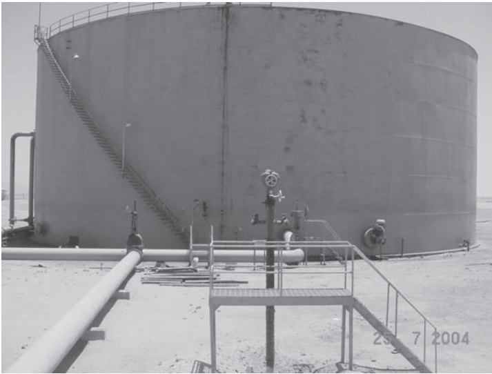
FIGURE 4.19a General tank view.
