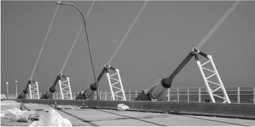
Figure 11.22 Cable-stay damping systems in Arthur Ravenel Jr. Bridge.
