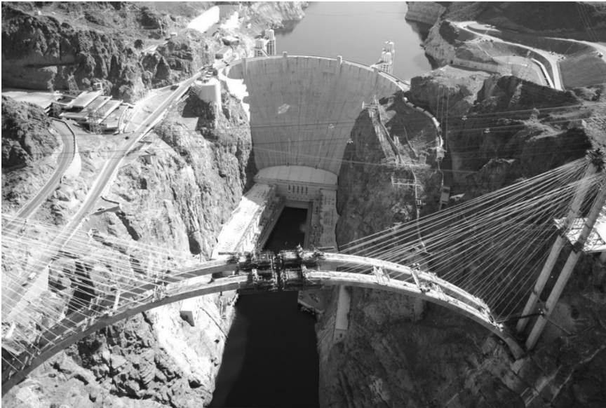
Figure 9.5 Cable-stayed segmental erecting of arch bridge. (Hoover Dam Bridge, Nevada, USA, Courtesy of galleryhip.com/hoover-dam-bridge-construction.html .)
