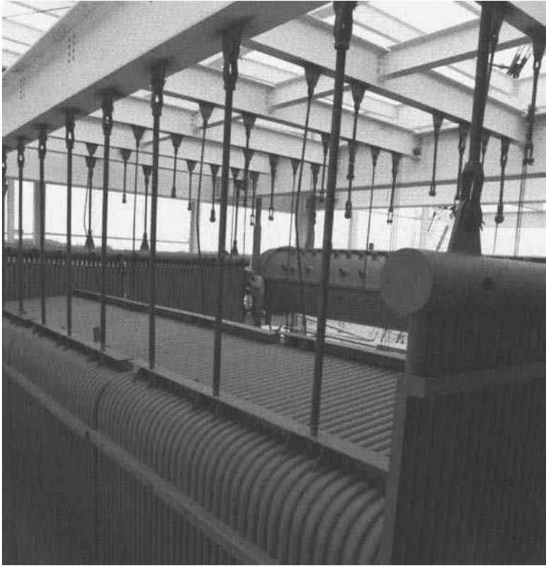
FIGURE 7.15 Top-suspension rods in an industrial boiler.
