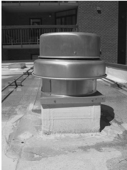
FIGURE 5-24 Photograph of a downflow exhaust fan.
