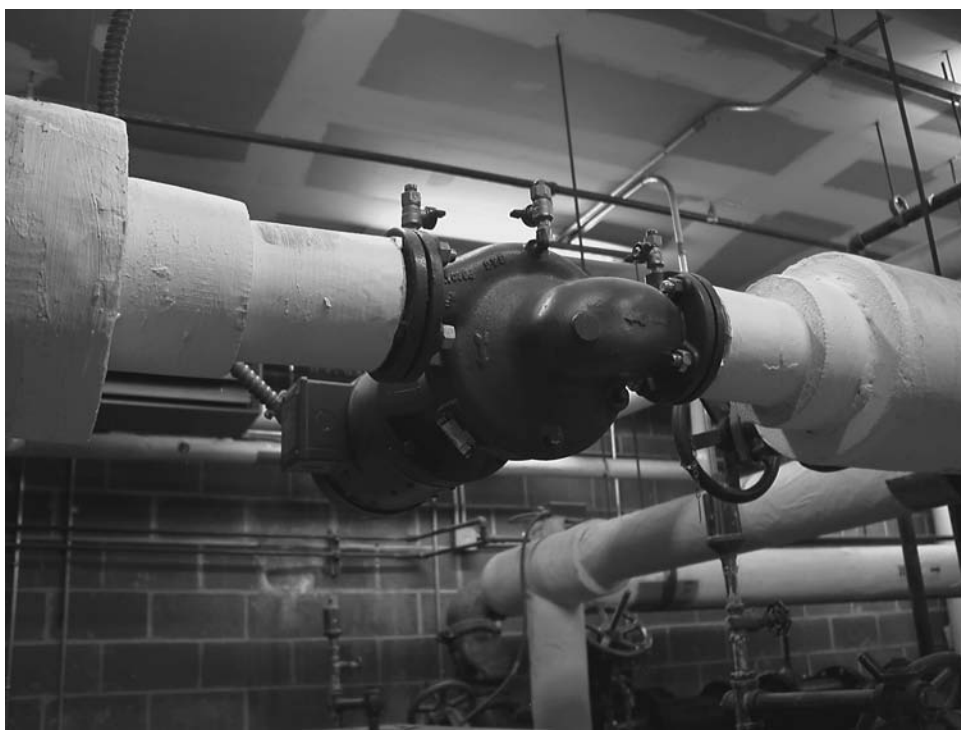
FIGURE 4-33 Photograph of an in-line pump.
