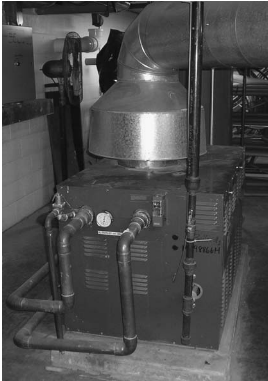
FIGURE 4-4 Photograph of a draft hood.
