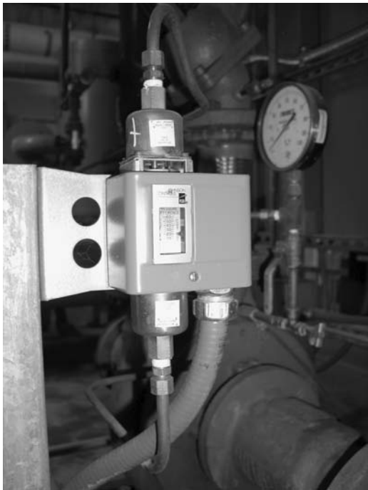
FIGURE 9-2 Photograph of a differential pressure switch.
