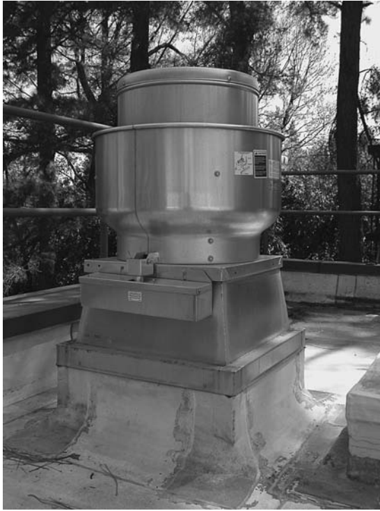
FIGURE 5-23 Photograph of an upblast grease exhaust fan.
