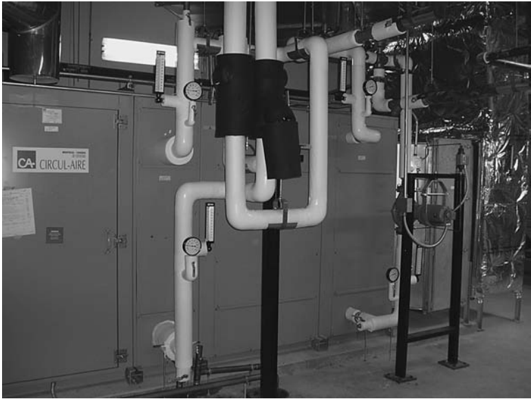
FIGURE 5-21 Photograph of a modular central station DOAS with a hot water heating coil, wrap-around heat pipe refrigerant coil, and a chilled water coil.
