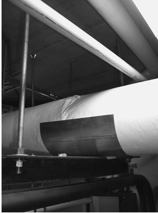
FIGURE 6-4 Photograph of a trapeze pipe hanger.
