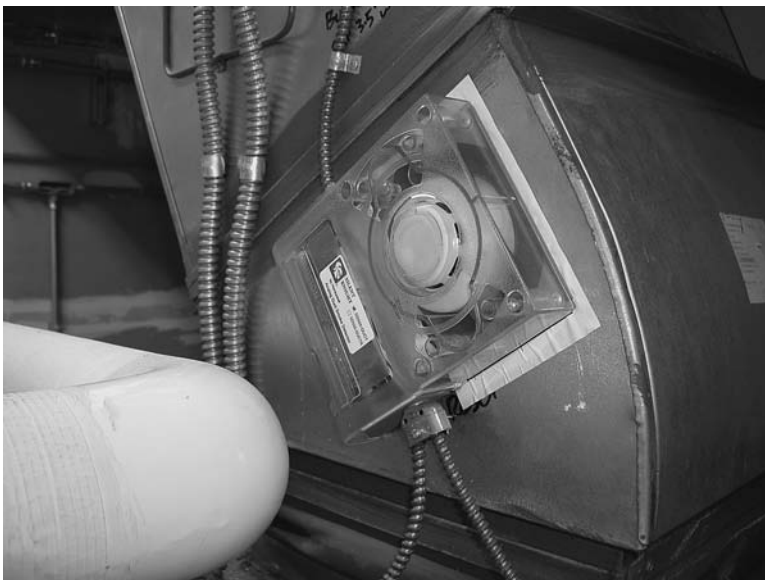
FIGURE 9-3 Photograph of a duct smoke detector.
