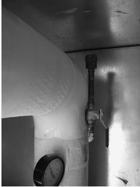
FIGURE 3-39 Photograph of a manual air vent.
