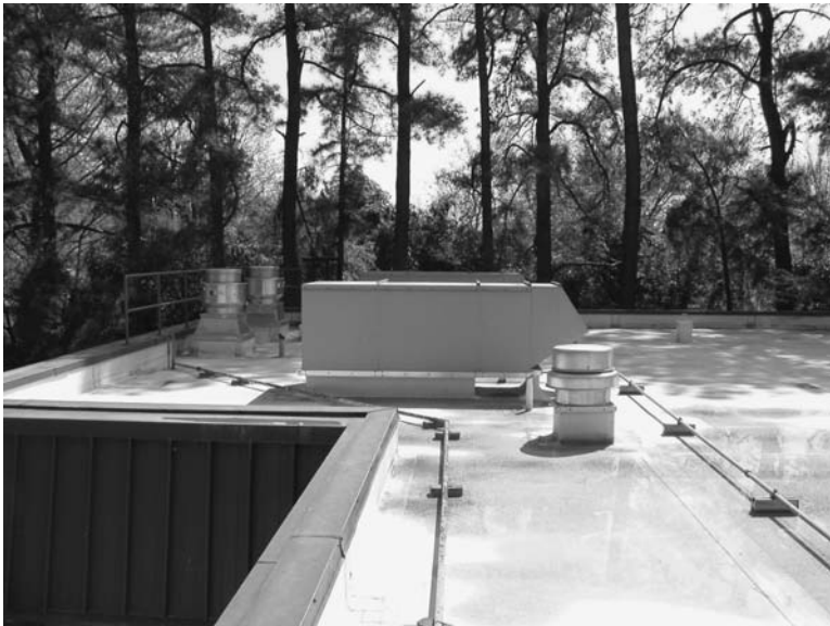
FIGURE 5-26 Photograph of two kitchen exhaust hood makeup air units with indirect gas-fired heaters, two upblast grease exhaust fans, and a downflow exhaust fan.
