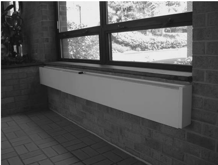
FIGURE 7-4 Photograph of a wall-mounted FTR with manual damper, which controls the airflow through the FTR.
