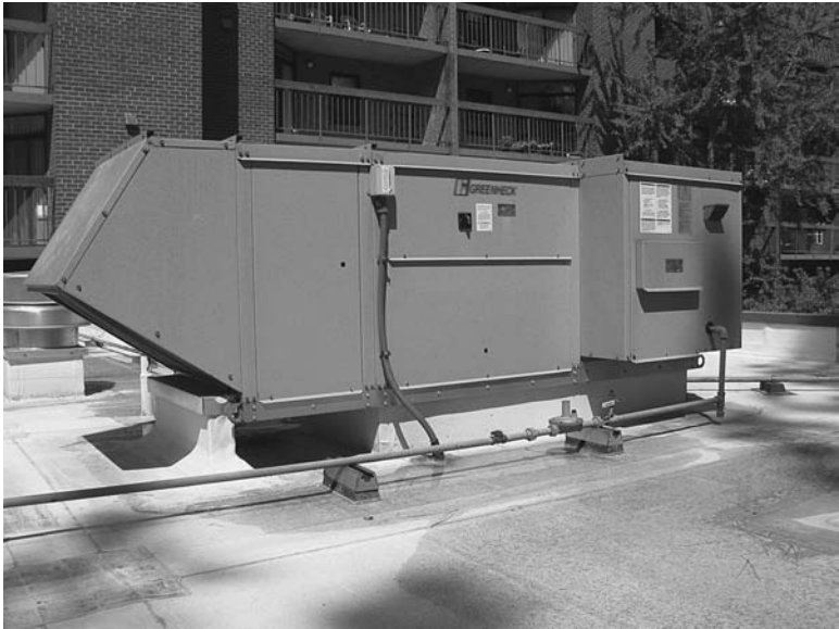
FIGURE 5-22 Photograph of a kitchen exhaust hood makeup air unit with an indirect gas-fired heater.
