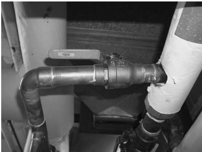
FIGURE 3-17 Photograph of a two-piece ball valve with solder ends—installed.
