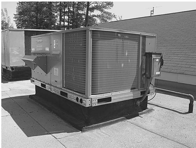
FIGURE 5-15 Photograph of a packaged RTU with indirect gas-fired heater and DX cooling coil.
