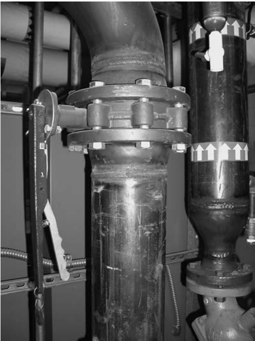
FIGURE 3-14 Photograph of a lug-style butterfly valve—installed.
