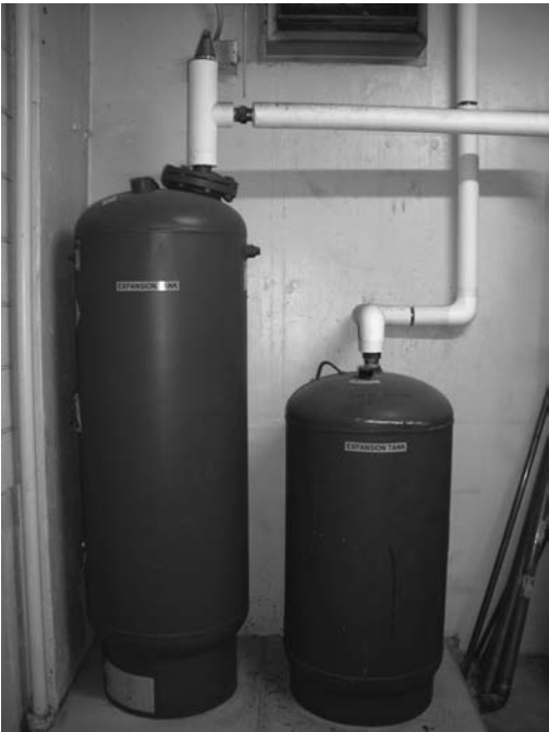
FIGURE 4-25 Photograph of an expansion tank.
