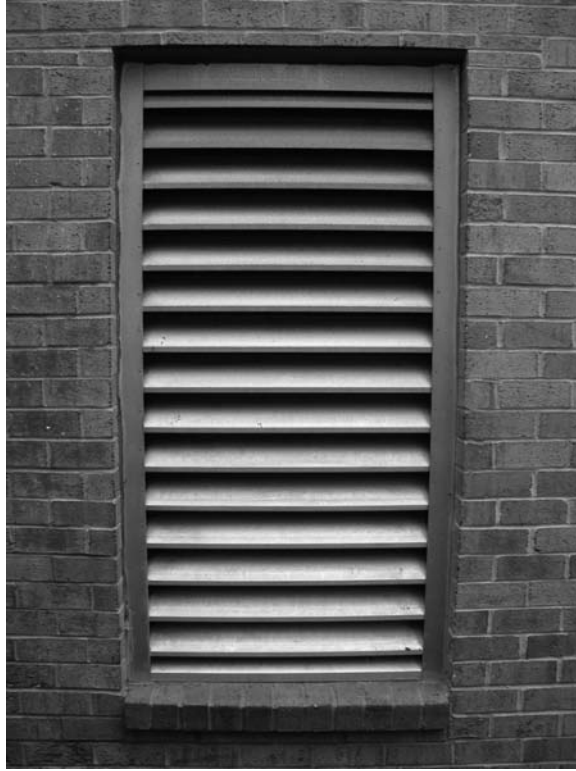
FIGURE 2-7 Typical wall louver.
