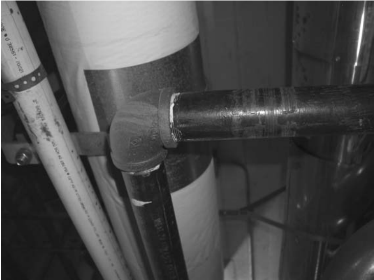
FIGURE 3-1 Photograph of a cast iron elbow with threaded ends.
