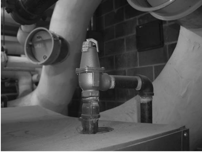
FIGURE 3-26 Photograph of a hot water pressure relief valve.
