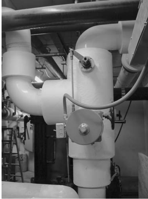
FIGURE 3-30 Photograph of linked butterfly valves used as a 3-way valve.
