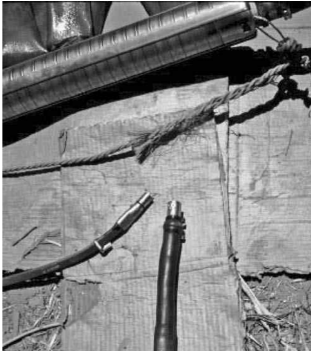
FIGURE 8.43 PV pump damaged cable splice where conductors have worn through from hauling the pump up and down on the pump cable rather than the security rope (Roatan, Honduras).
