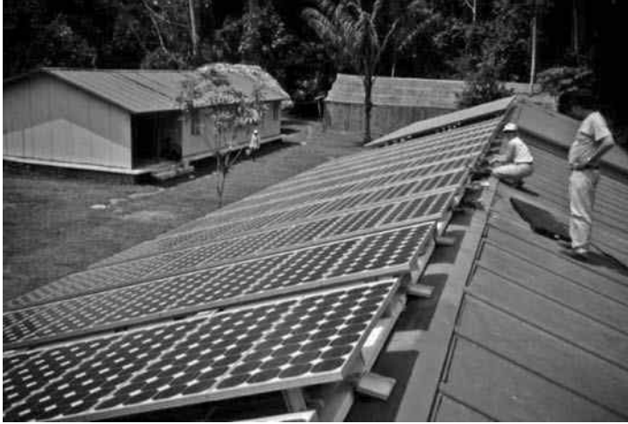
FIGURE 7.3 Mexico's first NEC -compliant PV system installed at Montes Azules Biosphere Reserve in Chiapas (1998) by WWF/USAID, Conдумex, Sandia, and NMSU.
