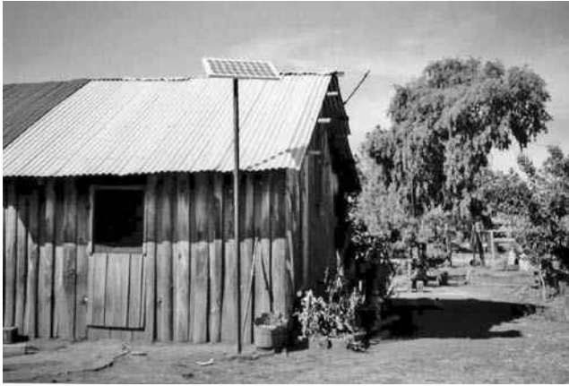
FIGURE 8.17 Solisto 50 W p PV lighting system installed in Talayotes, Moris County, Chihuahua.
