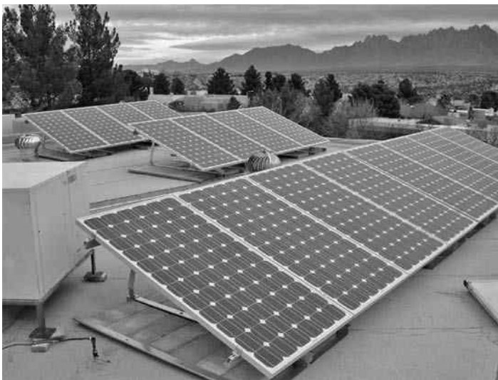
FIGURE 6.8 PV modules tilted to maximize annual energy production for utility interactive residential installation in Las Cruces, New Mexico.
