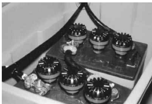
FIGURE 11.11 Catalytic recombiner caps used on deep-cycle LA batteries for a PV system. Note the rubber container to contain any possible acid spills and appropriate battery cables.
