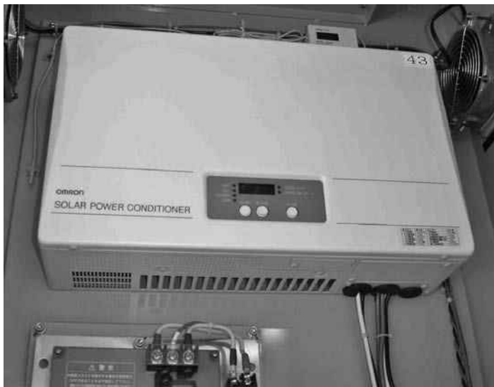
FIGURE 8.9 Four-kiloWatt transformerless Omron inverter on AIST PV parking structure.
