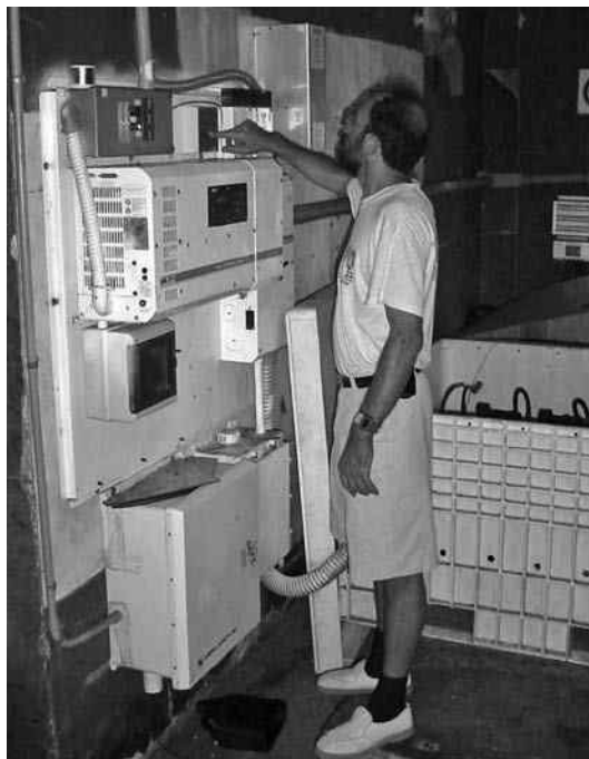
FIGURE 8.25 Isla Contoy solar and wind energy power center, inverter, controls, and batteries.
