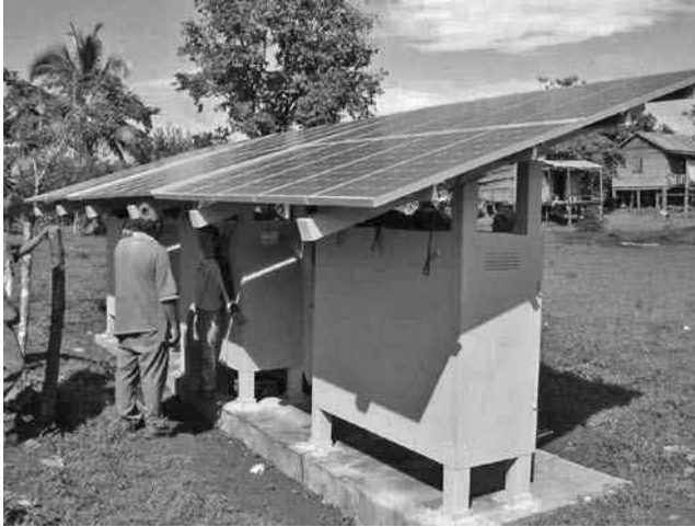
FIGURE 8.19 One of the three PV battery charging stations (NW system) at Francia Sirpi, Nicaragua.
