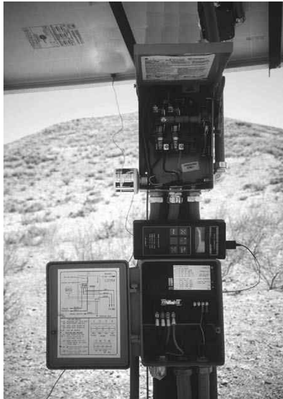
FIGURE 8.39 Typical pump controller with overcurrent protection for PV water-pumping system in Chihuahua, Mexico.
