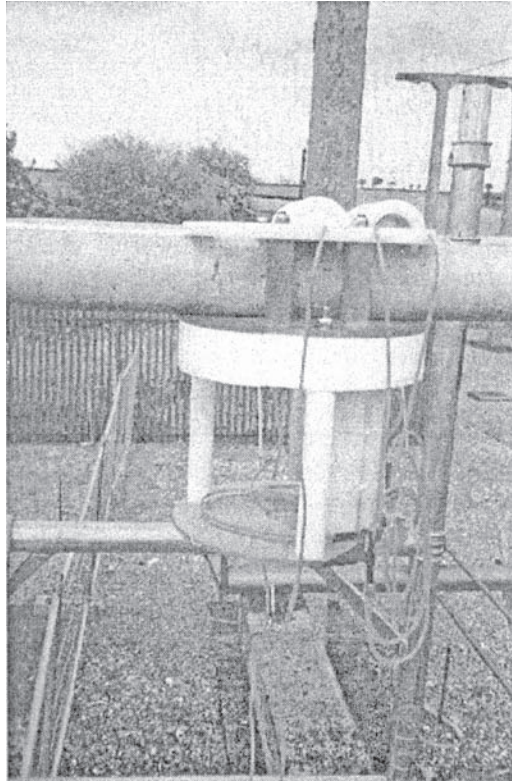
FIGURE 3.34 Close-up of the OCT/OVT installation.
