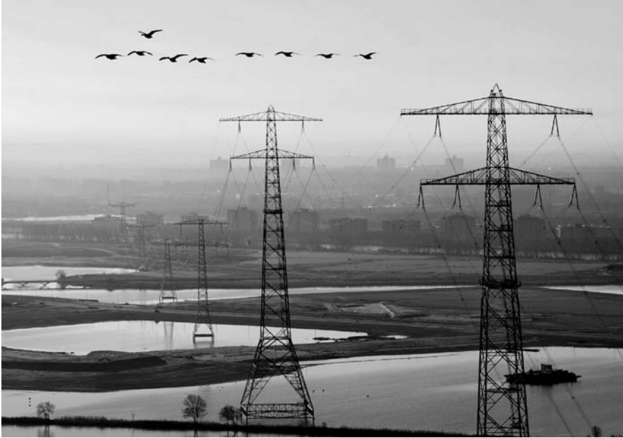
Figure 3.28 Overhead transmission lines. Reproduced by permission of TenneT TSO B.V.
