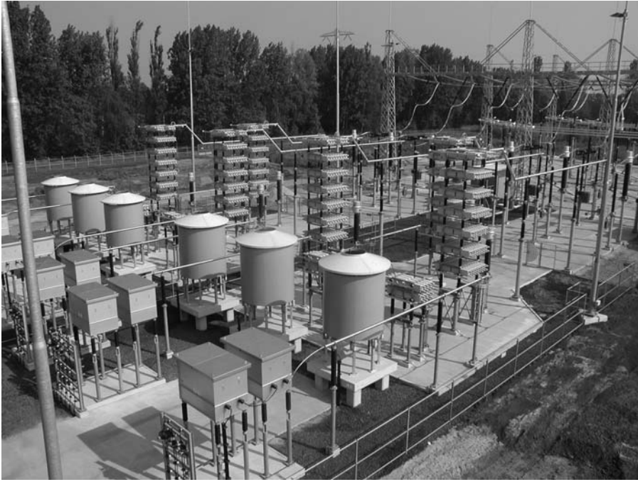
Figure 5.14 Capacitor banks. Reproduced by permission of TenneT TSO B.V.
