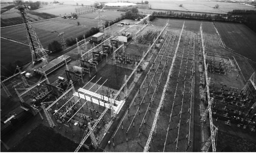
Figure 3.7 An open-air substation. Reproduced by permission of TenneT TSO B.V.
