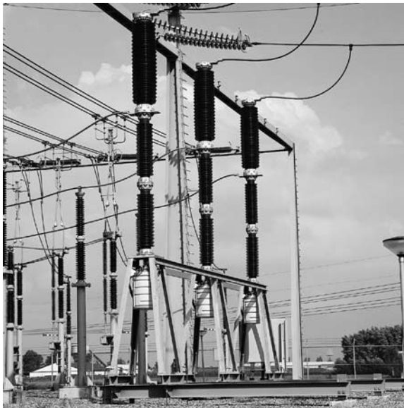
Figure 3.8 Three single-phase circuit breakers. Reproduced by permission of TenneT TSO B.V.
