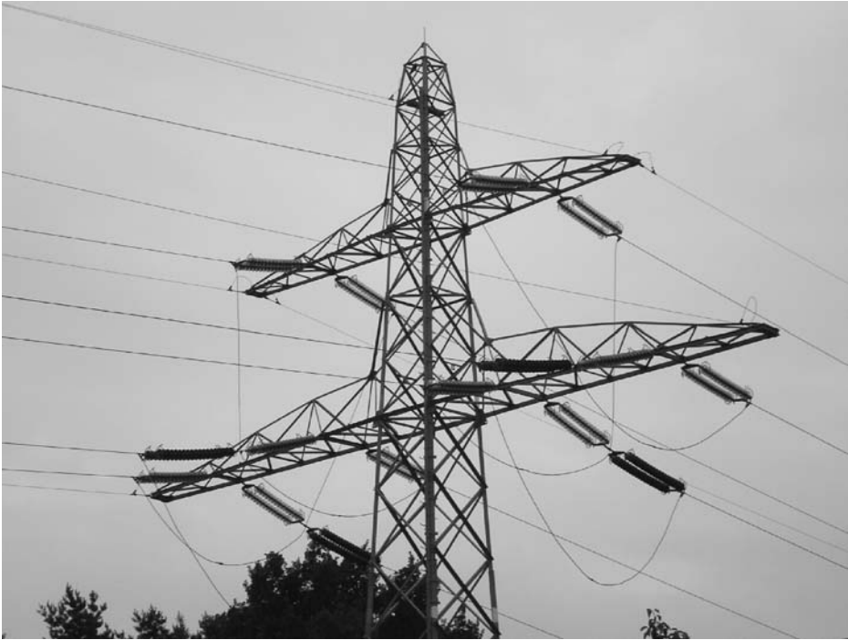
Figure 3.47 A twisting pylon.
