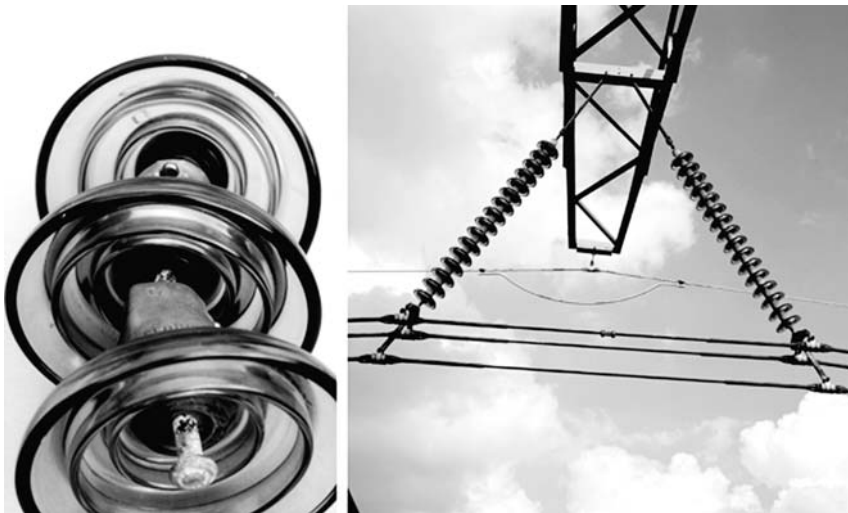
Figure 3.32 Three discs of an insulator string and a three-conductor bundle suspended from a tower by an insulator string. Reproduced by permission of TenneT TSO B.V.
