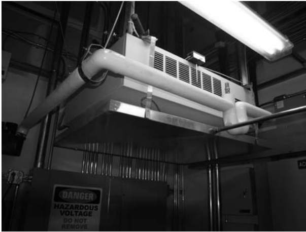
FIGURE 40.10 Secondary drain pan. (Photo by author, courtesy of Hathaway Dinwiddie Construction Company and The University of Southern California.)
