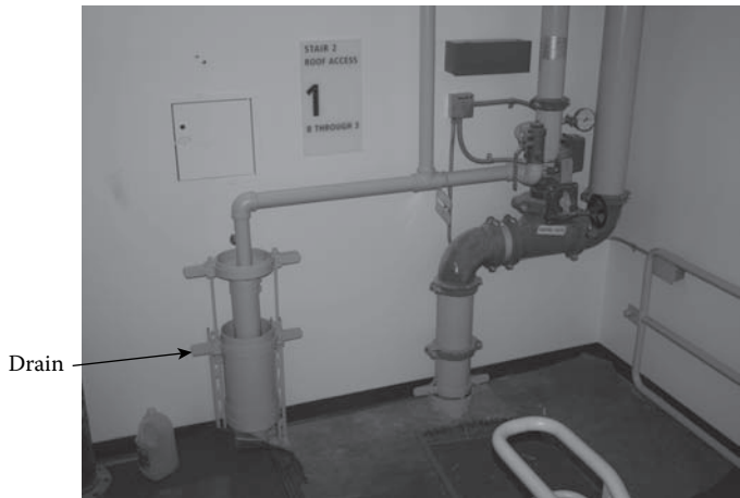
FIGURE 38.5 Fire sprinkler drain. (Photo by author, courtesy of Hathaway Dinwiddie Construction Company and The California Institute of Technology.)
