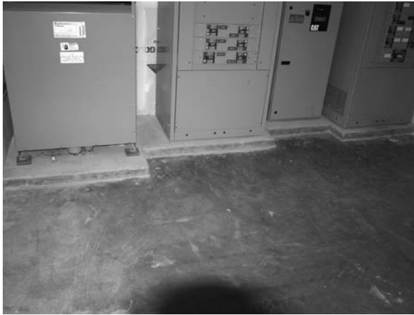
FIGURE 6.2 Housekeeping (equipment) pad. (Photo by author, courtesy of The University of Southern California.)
