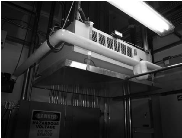
FIGURE 21.4 Secondary drain pan. (Photo by author, courtesy of Hathaway Dinwiddie Construction Company and The University of Southern California.)
