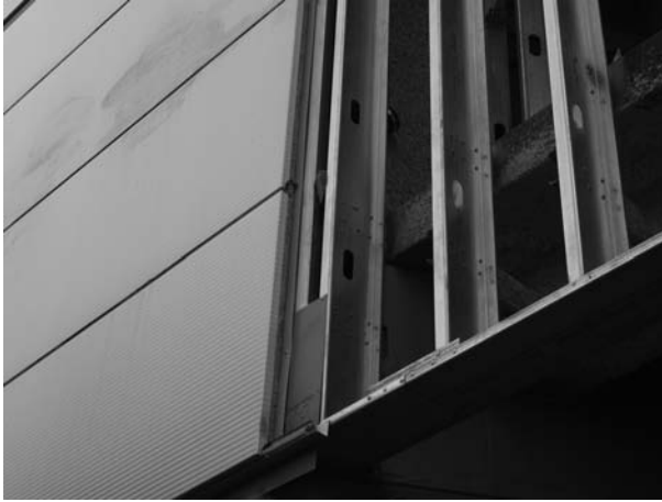
FIGURE 19.2 Metal panels. (Photo by author, courtesy of Hathaway Dinwiddie Construction Company and California State University Northridge.)
