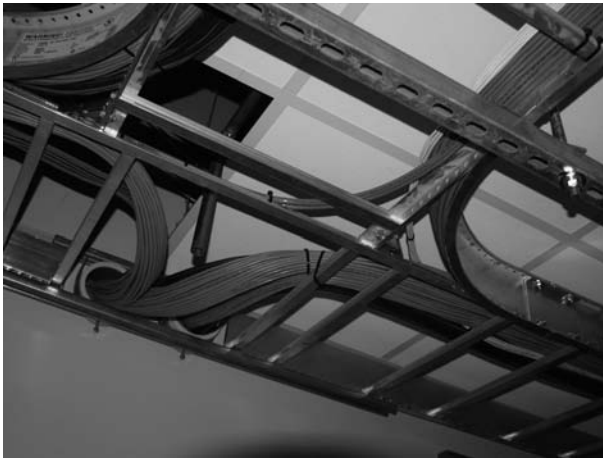
FIGURE 41.8 Cable tray. (Photo by author, courtesy of Hathaway Dinwiddie Construction Company and The University of Southern California.)
