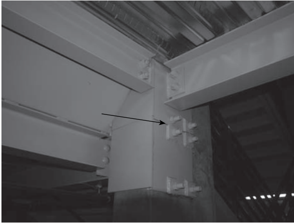
FIGURE 47.1 Surface-mounted steel brackets necessary due to missed embeds.
