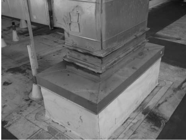
FIGURE 40.9 Duct flashing at roof. (Photo by author, courtesy of The University of Southern California.)
