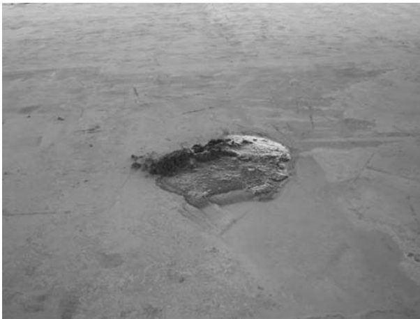
FIGURE 7.5 Concrete seepage from concrete placement above.
