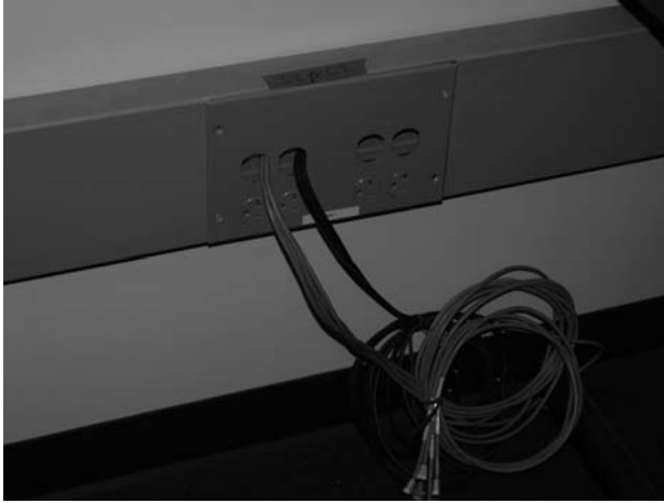
FIGURE 41.7 Wiremold. (Photo by author, courtesy of Hathaway Dinwiddie Construction Company and The University of Southern California.)
