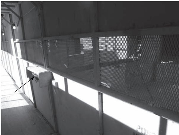
FIGURE 39.5 Temporary fire department connection.
