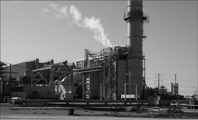
6.6: Midlothian, TX, USA: GT24 single-shaft combined cycle block with once through heat recovery boiler. One of six units on the site near Dallas, TX.
