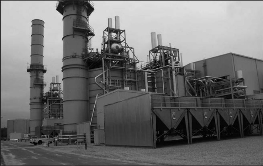
6.4: Blackstone, MA, USA: American National Power's standard GT24 single shaft block with Benson boilers including SCR units for ultra-low NO x output.
