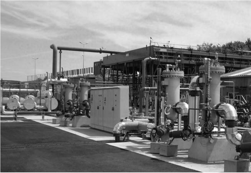
7.4: Soultz sur Foret, France. Water at 200^{\circ}\text{C} is pumped from 5000 m below site to a heat exchanger with isobutane driving the turbine. (Photo courtesy of GEIE EMC)
