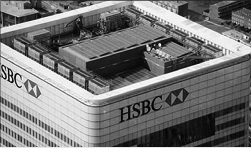
8.1: London, UK: HSBC has installed this photovoltaic array on their headquarters' roof which is expected to generate 77 500 kWh per year. (Photo courtesy of HSBC)
