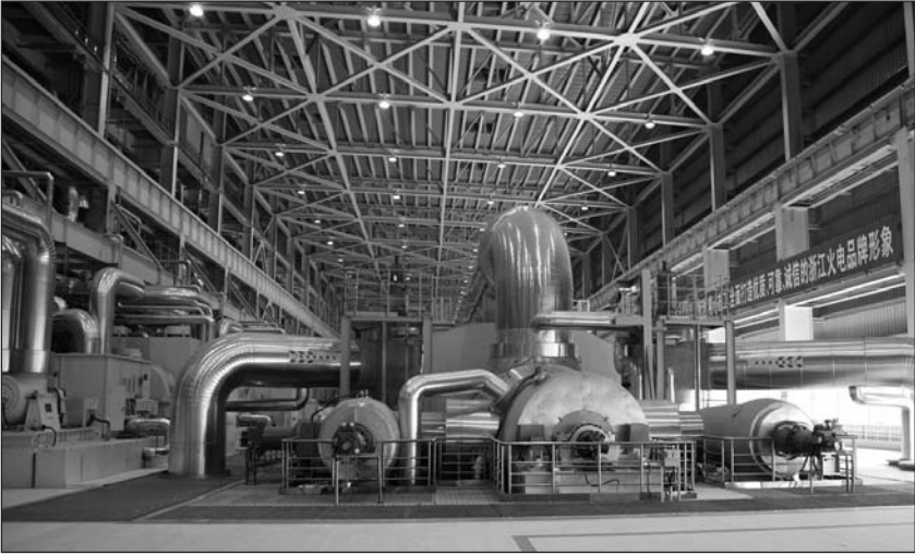
4.3: Zhejiang, China: One of four 1000 MW supercritical steam turbines in the Yuhuan power station of Huaneng Power Inc. (Photo courtesy of Siemens)
