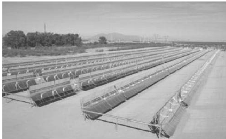
Figure 1 APS Saguaro Solar Trough Power Plant. Source: Courtesy of Arizona Public Service (APS).
