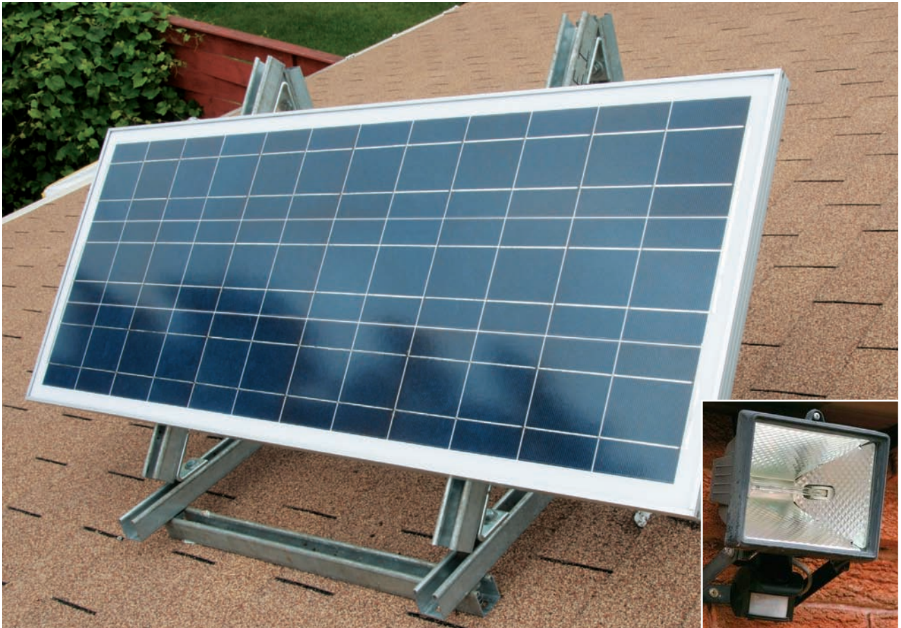
This 60-watt solar panel is mounted on a garage roof and powers a self-contained home security lighting system. Not only does this save energy costs, it keeps the security lights working even during power outages.
