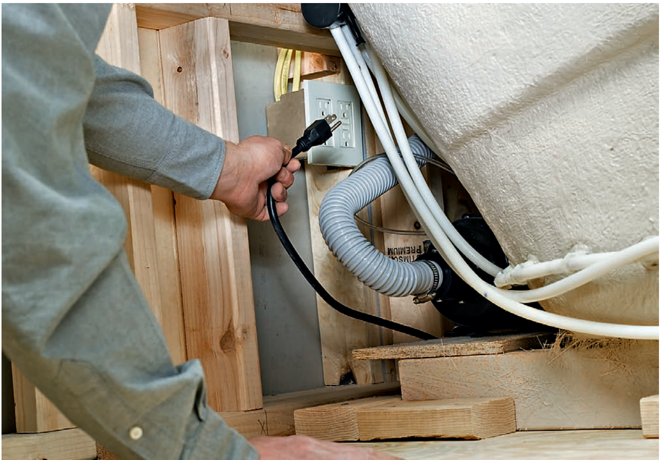
Receptacles for whirlpool tubs must be GFCI protected.
