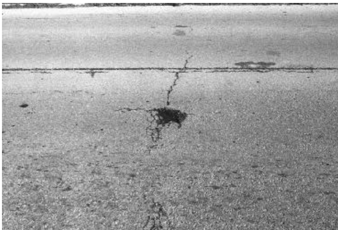
FIGURE 3.33 Example of small pothole in flexible pavement.
