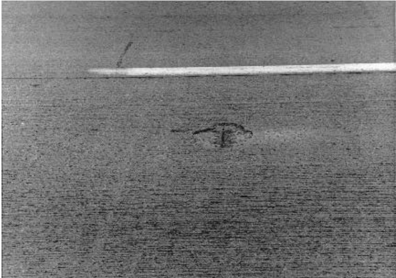
FIGURE 3.23 Example of popout in jointed rigid pavement.
