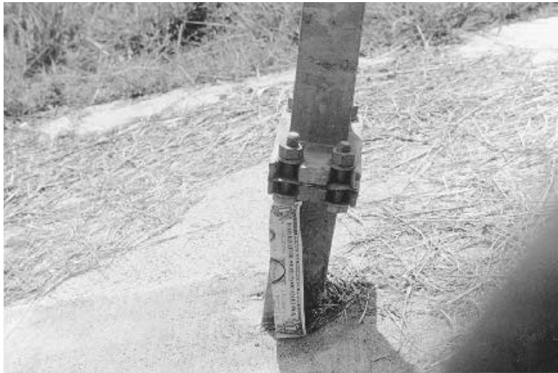
FIGURE 7.52 Improper installation of slip base anchor piece.
