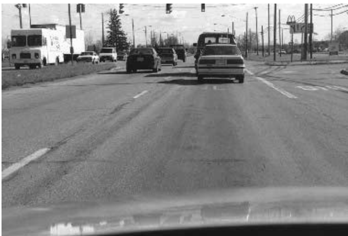
FIGURE 3.34 Example of rutting in flexible pavement.
