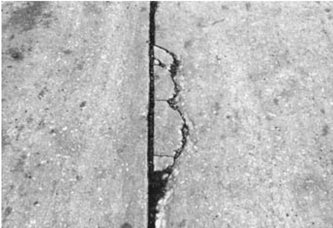
FIGURE 3.25 Example of joint spalling in rigid pavement.
