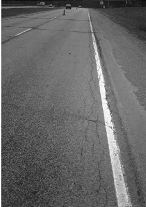
FIGURE 3.40 Example of edge cracking in flexible pavement.
