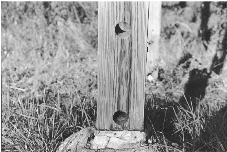
FIGURE 7.62 Weakened wooden post for multiple supports.
