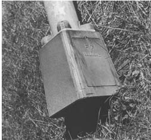
FIGURE 7.96 Separation of bottom flange from T-base.
