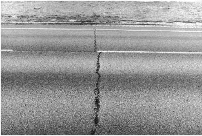
FIGURE 3.37 Example of transverse cracking in flexible pavement.
