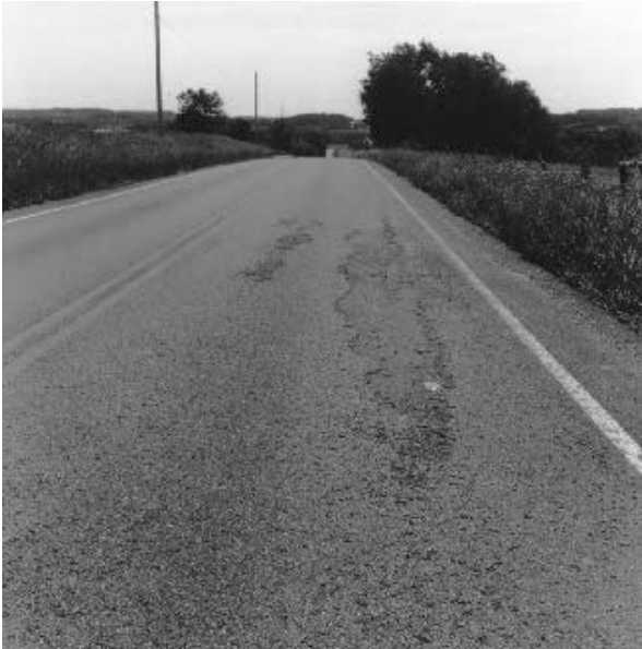
FIGURE 3.31 Example of raveling in flexible pavement.
