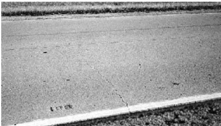
FIGURE 3.55 Hairline crack in rigid pavement.
