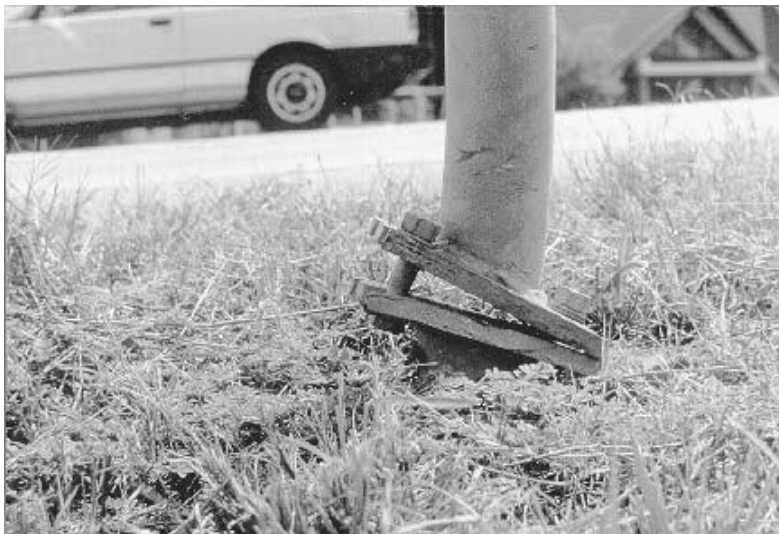
FIGURE 7.26 Loose slip base caused by vibration.
