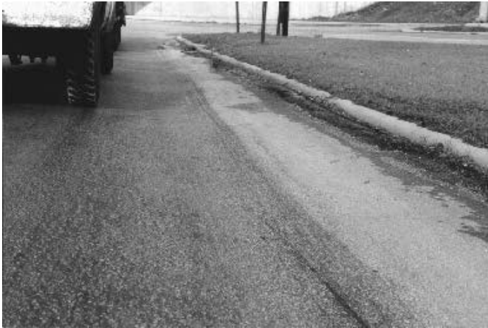
FIGURE 3.35 Example of corrugations in flexible pavement.
