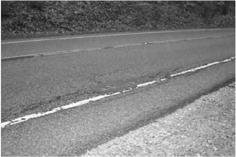
FIGURE 3.57 Localized wheel track and edge cracking.
