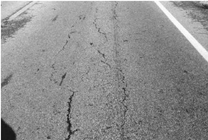
FIGURE 3.36 Example of longitudinal cracking in flexible pavement.
