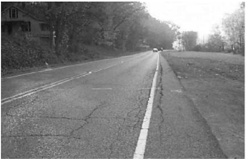
FIGURE 3.58 Localized edge cracking.
