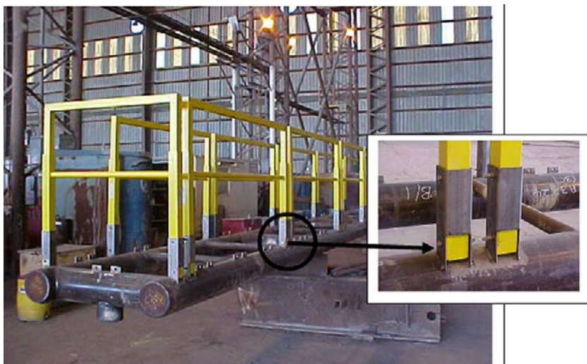
FIGURE 7.45 Handrail made from glass fiber-reinforced polymer (GFRP).
