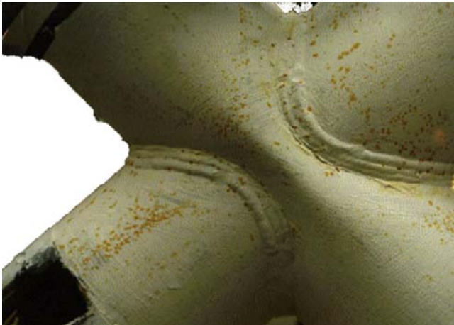
FIGURE 3.36 Buckling of the tubular joint.
