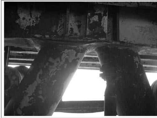
FIGURE 7.10 Fire-related effects on the main truss.
