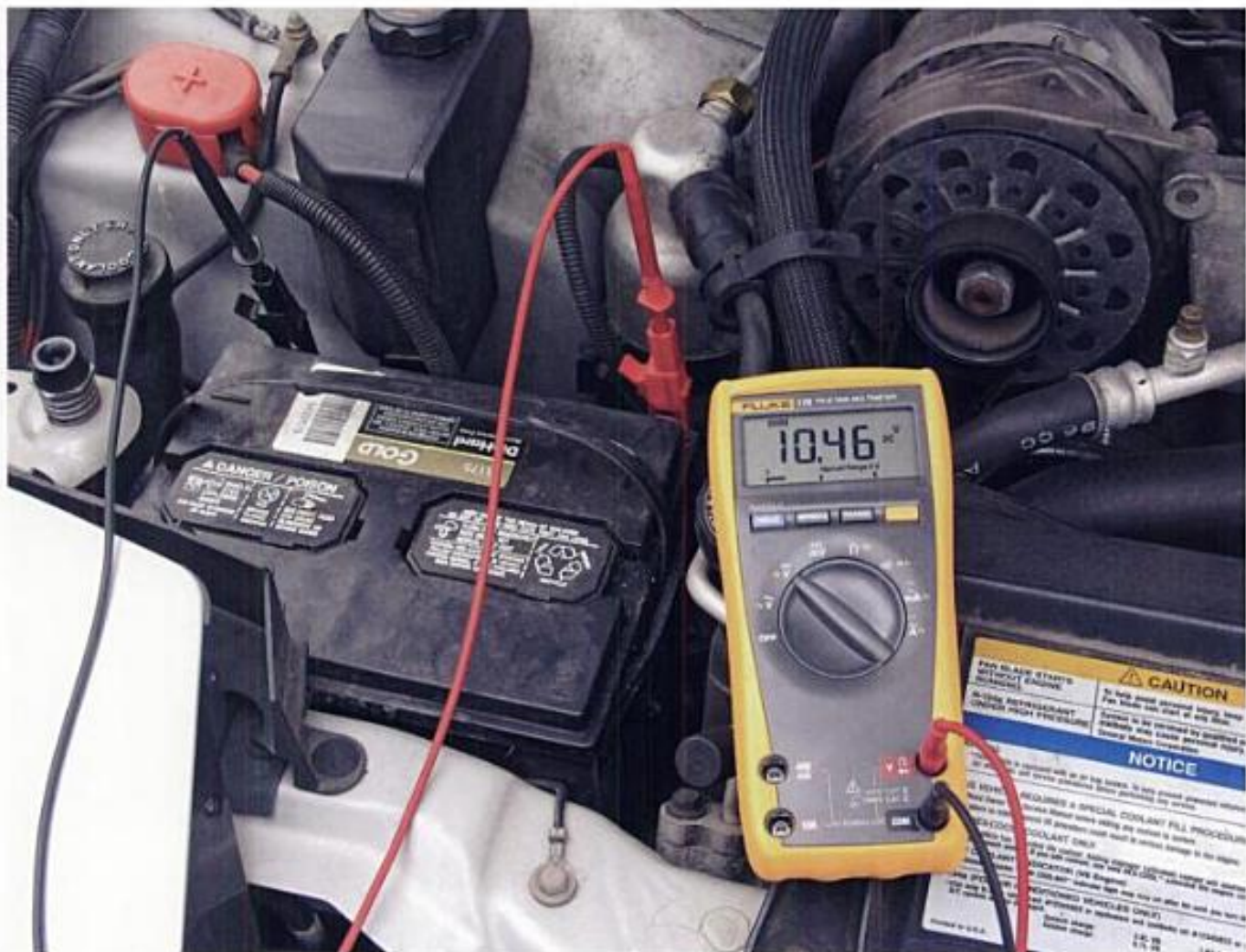
After cranking the engine for 10 seconds and with the starter still cranking, this battery is showing 10.46 volts, which indicates that it is in good condition.
