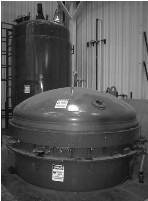
FIGURE 4.36 VPI tank used for large electric motors.
