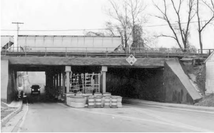
FIGURE 5.9 View of the restored wing wall, girder, and the abutment walls (East Street Viaduct, West Virginia).
