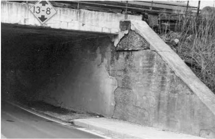
FIGURE 5.4 View of the damaged wing wall (East Street Viaduct, West Virginia).
