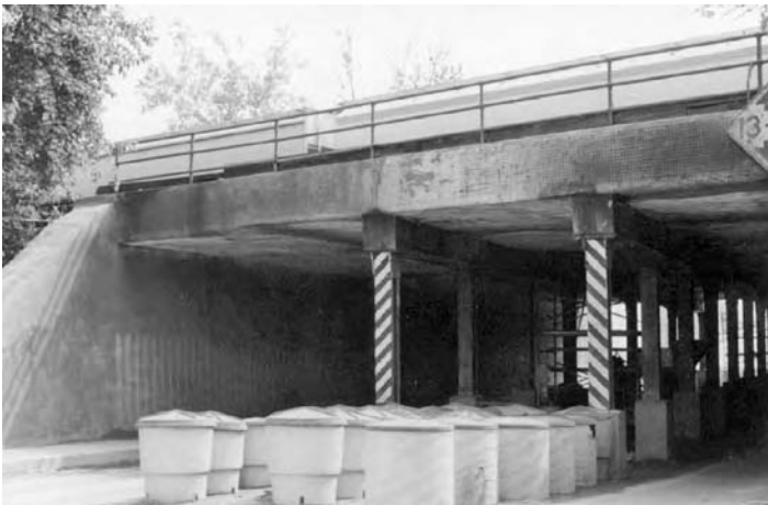
FIGURE 5.6 Wing wall and abutment being restored with GFRP (East Street Viaduct, West Virginia).
