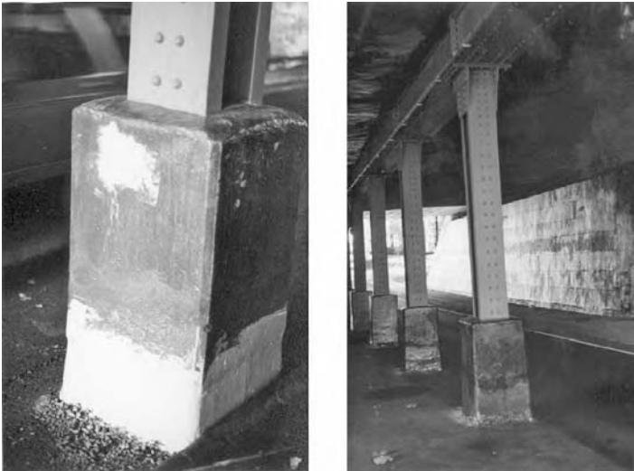
FIGURE 5.8 Concrete pedestals pretreated (left) and wrapped with a FRP fabric (right) (East Street Viaduct, West Virginia).
