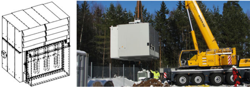
Fig. 4 Enclosure for outdoors ( left ). Unloading of HiDry 72 (16 MVA) with the enclosure ( right )
