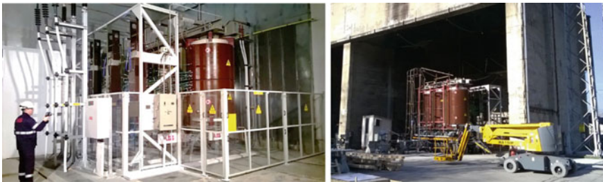
Fig. 7 HiDry 72 (34 MVA) installed in the substation ( left ). One of the units 34 MVA was withstand short-circuit tested in CESI (Milan, 2014)
