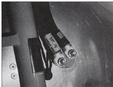
Battery cables were fabricated for this installation. Note permanent labels installed on them. These heavy wires lead to master cutoff switch on opposite side of panel.
