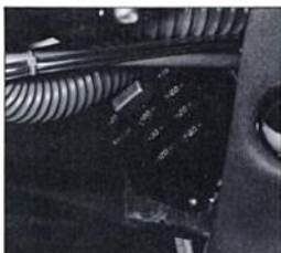
This fuse panel is located under instrument panel next to driver's right knee, where there was plenty of room for panel and associated wiring. It is easily accessible, close to electrical distribution panel (terminal strips with 92 connections), and protected from accidental contact by moving parts.
