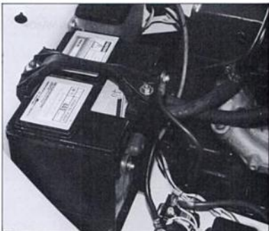
This battery location was dictated by two factors. First, the fiberglass body was molded with battery shelf in place. Second, this location places battery within about 18 inches of starter motor, minimizing cable length.
