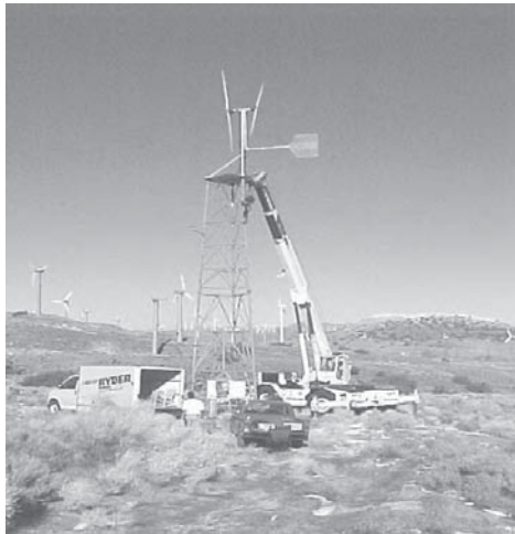
FIGURE 19.19 Contrarotating turbine installation on a 50-ft tower at Oak Creek Energy Systems test site in Mojave, CA.
