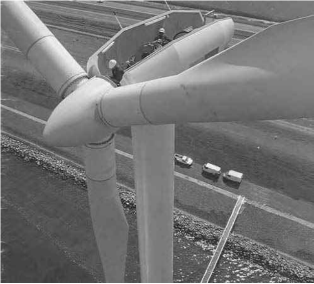
FIGURE 4.3 A large nacelle under installation. (From Nordtank Energy Group, Denmark. With permission.)
