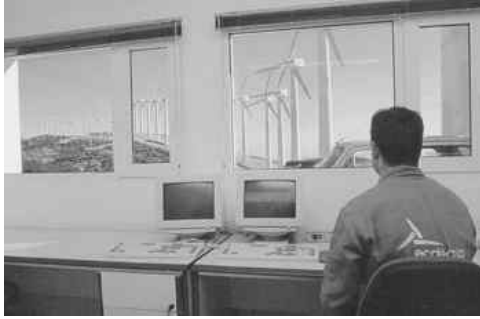
FIGURE 4.1 Baix Ebre wind farm and control center, Catalonia, Spain. (From Wind Directions , Magazine of the European Wind Energy Association, London, October 1997. With permission.)
