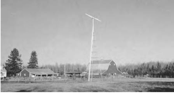
FIGURE 12.5 Remote farms are a major market for the stand-alone power systems. (From World Power Technologies, Duluth, MN. With permission.)
