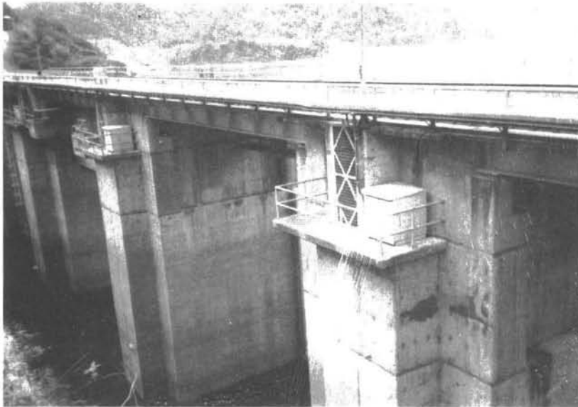
Fig. 3.16 The gating system where water from the dam flows through 4 inlets.
