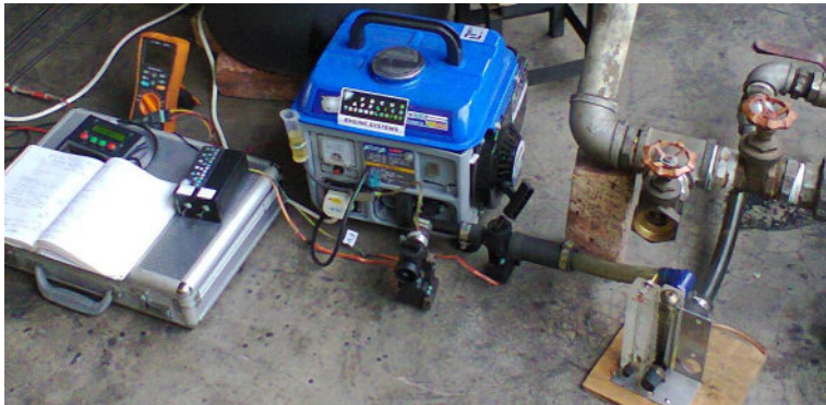
Figure 11. AFR and throttle controller are to the left of the engine, as is the digital display. Note that the gas supply system has relatively large pipes to supply the unpressurized syngas.
