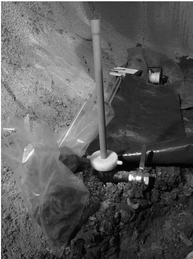
Figure 8.44 Well used as a piezometer. (Photo Credit: Crossrail Ltd., used with permission.)
