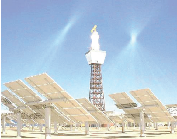
Figure 7.7. Solar thermal plant.
