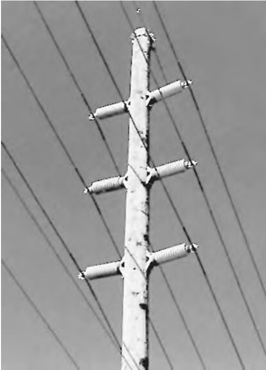
FIGURE 10.2 69-kV transmission line with post insulators.
