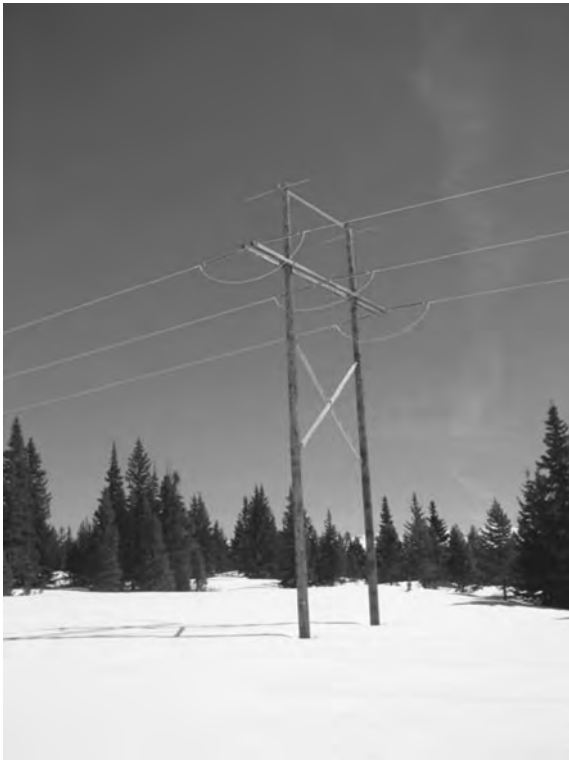
FIGURE 19.1 220 kV line with H-frame wooden towers.
