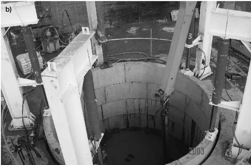
Figure 4.27 a) Caisson-sinking method to construct shafts (after BTS/ICE 2004, used with permission from Thomas Telford Ltd), b) shows the construction of a reception shaft for a pipe jacking operation as part of the Terminal 5 project at Heathrow, UK
