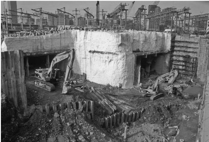
Figure 5.79 Breakthrough of two of the jacked tunnels, showing the freezing operation at the ground surface (courtesy of Massachusetts Turnpike Authority)
