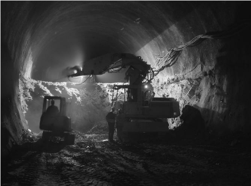
Figure 5.47 Example of a NATM crown and bench excavation during the construction of the Katschberg Tunnel, Austria
