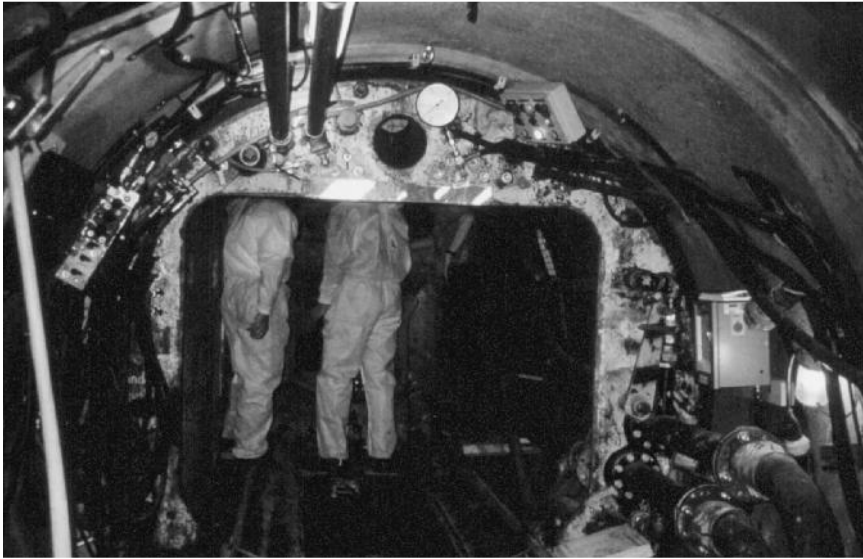
Figure 4.16 Airlock arrangement on a pipe jacking project for a new sewer in Germany (see section 5.11 for a description of pipe jacking)
