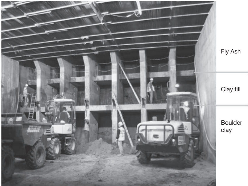
Figure 5.74 Rear view of the cellular reinforced concrete shield (annotation indicates the ground strata) (Allenby and Ropkins 2004, courtesy of BAM Nuttall Ltd and John Ropkins Ltd)
