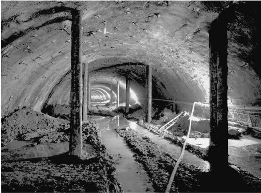
Figure 7.25 Emergency support measures using tree trunks during the tunnel excavation (Eggetunnel, crown heading) (courtesy of Professor Dr-Ing. habil. Reinhard B. Rokahr, photograph by Ulrich Mertens DFA DGPh, Atelier für Kunst und Fotografie, Hamburg)
