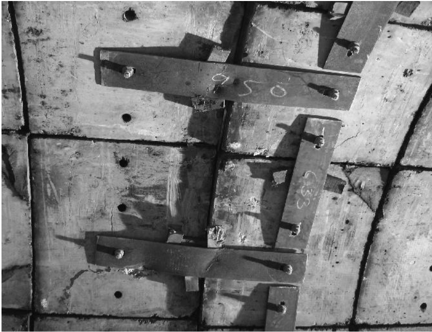
Figure 8.16 Existing Piccadilly Line Westbound Tunnel showing steps of up to 60 mm between concrete segments
