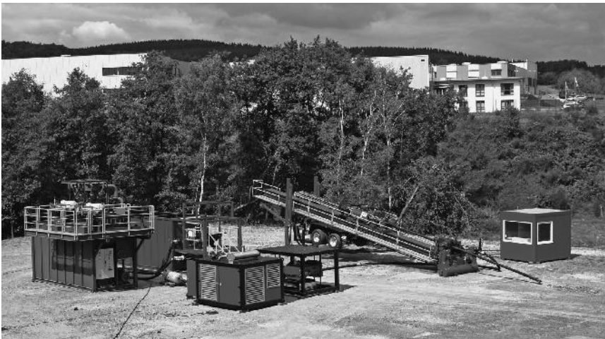
Figure 5.88 Example of a large HDD rig and associated facilities, pumps and mud recirculation system (courtesy of Prime Drilling HDD-Technology)
