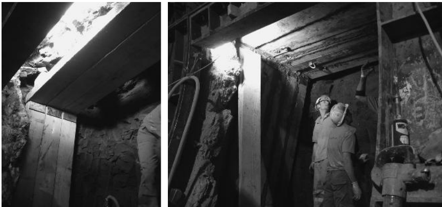
Figure 5.1 Timber heading as used in London Clay for constructing a connecting passage between two other tunnels (approximately 30–80 m 2 ), King's Cross Station upgrade, London (construction period 2002–2008) (courtesy of ALPINE BeMo Tunnelling GmbH Innsbruck)
