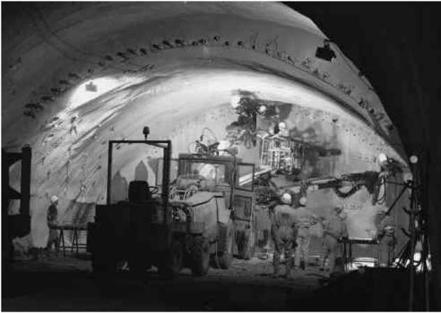
Figure 4.14 Forepoling using dowels as a roof pipe umbrella on the Lainzer Tunnel LT31 in Vienna, Austria
