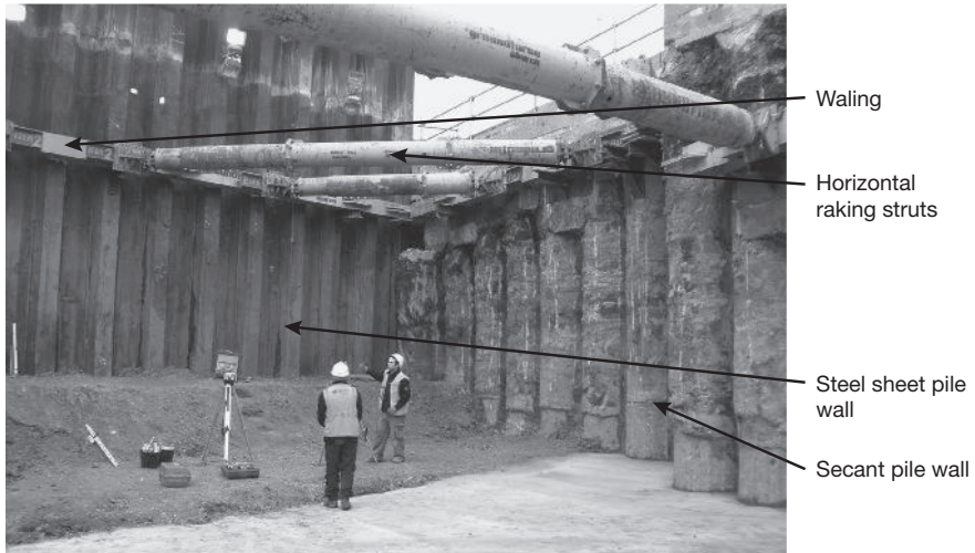
Figure 5.59 Secant pile wall as used as part of the jacking pit for a jacked box tunnel at Owen Street, Tipton, UK (see section 5.10 on jacked box tunnels). The photograph also shows the steel sheet pile headwall with its waling and horizontally raking struts transferring the headwall loading into one of the secant piled sidewalls (courtesy of BAM Nuttall Ltd and John Ropkins Ltd)
