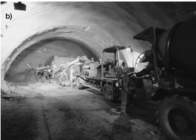
Figure 4.19 a) Manual spraying and b) Spraying equipment used during the construction of the Lainzer Tunnel LT31 in Vienna, Austria
