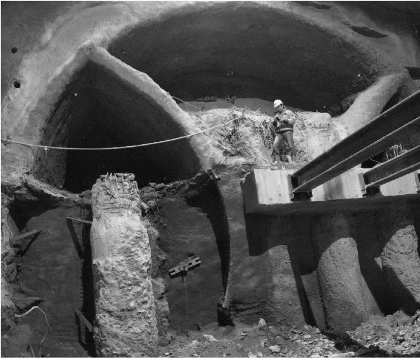
Figure 8.19 Crown excavated, and enlargement of leading side wall drift started. Remaining bracing still in place
