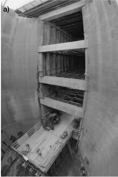
Figure 8.18 a) Shaft 'Klimtgasse'. Excavation platform with planking nearly finished, b) excavation platform. Shoring towers in place, web girders are laid close together and covered in planking
