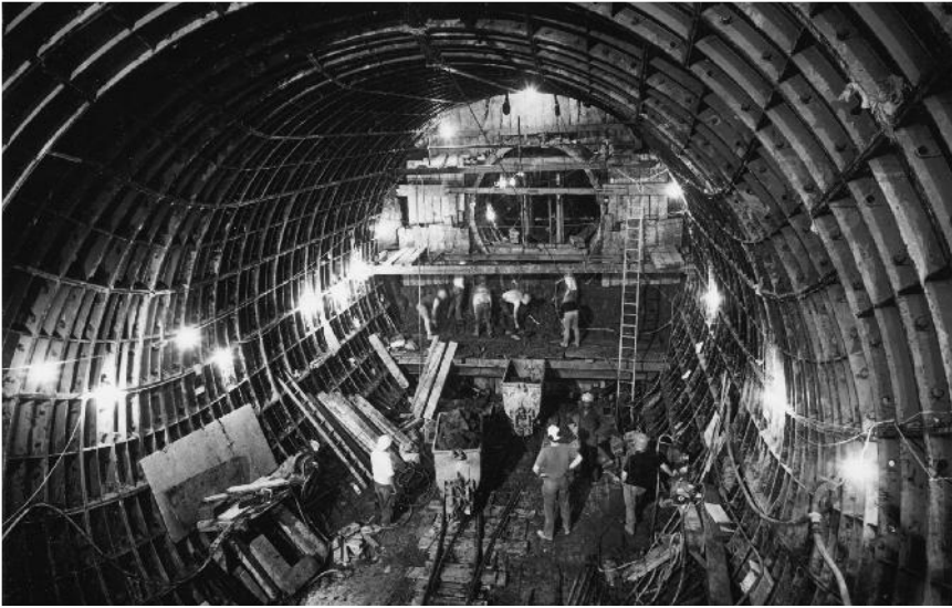
Figure 5.2 Construction of an escalator tunnel at The Angel Islington Station, London Underground, UK (completed in 1990). The tunnel was constructed at an angle of 30^\circ to the horizontal and used a pilot bore (3.7 m in diameter), which was then enlarged to the final diameter of 7.5 m (courtesy and copyright London Underground)
