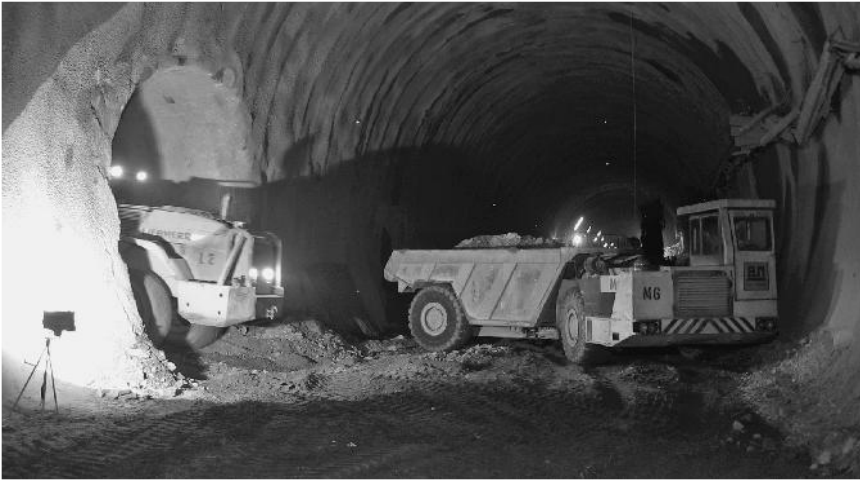
Figure 5.49 Example of mucking equipment used during the construction of one of the emergency cross passages of the Katschberg Tunnel, Austria
