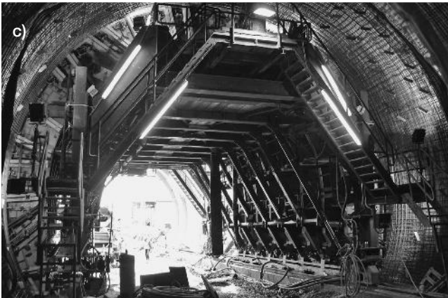
Figure 4.28 Construction of the inner lining, Heidkopf Tunnel, Germany, a) and b) setting up the shuttering at the tunnel portal, c) shuttering in the main tunnel
