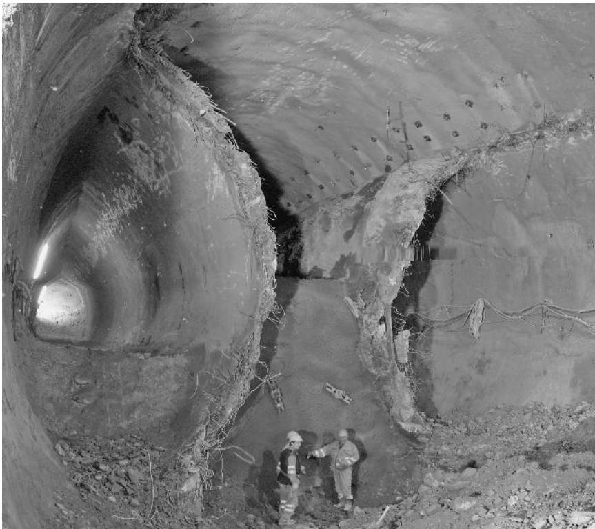
Figure 8.23 Construction of the invert at the total cross section (excavation Kern2 and demolition of inner walls of side wall drift)
