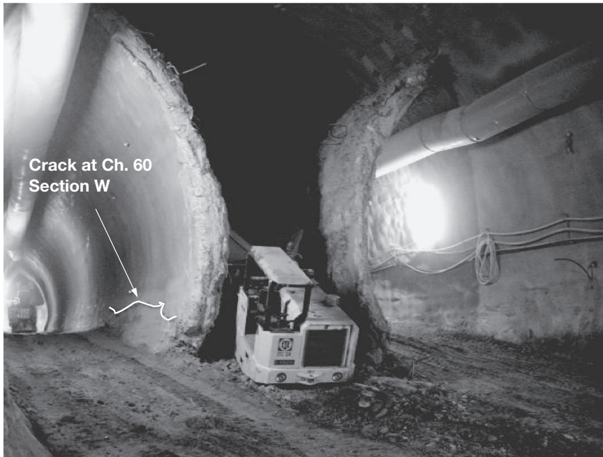
Figure 8.24 Crack in the inner wall of the side wall drift, section W, Chainage 52–60
