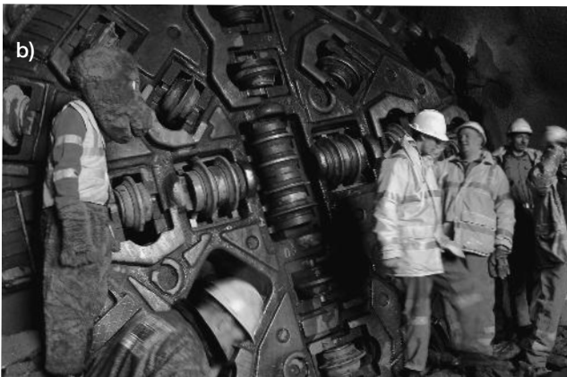
Figure 5.18 a) and b) 5.03 m diameter Herrenknecht S-351 Gripper TBM used at Glendoe, UK (courtesy of Herrenknecht)
