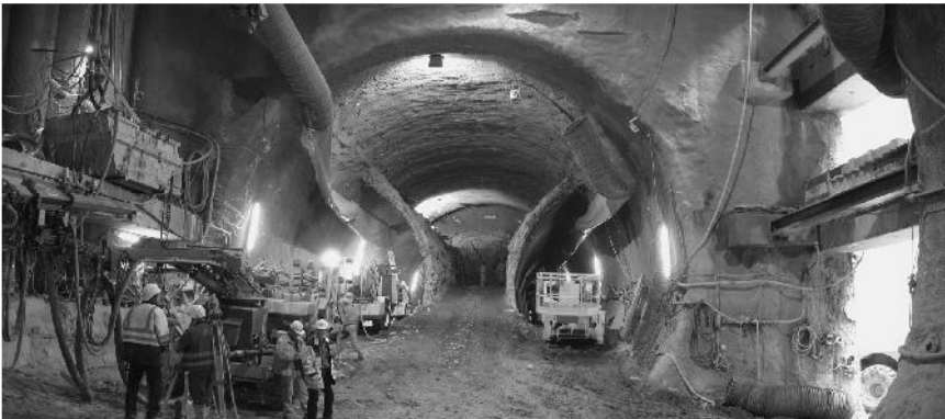
Figure 8.20 30 m of total cross section (on the RHS, the open oval section, the remainder of the lower most bracing can be seen still in place)
