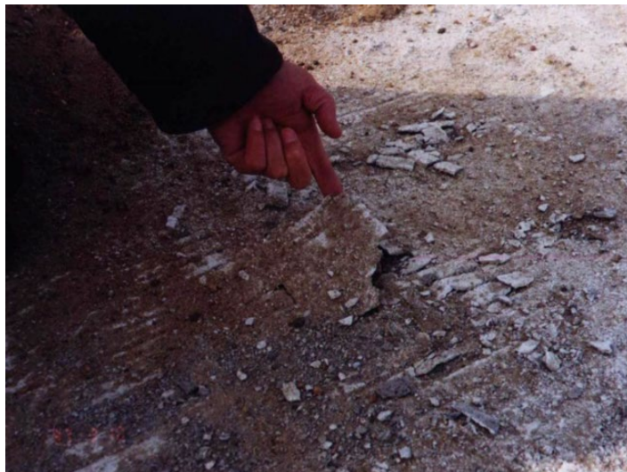
Figure 3.2 Salt scaling of concrete surface on road pavement in a cold region in China. Source: courtesy of Weizu Qin.
