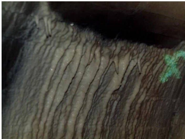
Figure 4.1 Speleothems ( \text{CaCO}_3 ) formed on the internal wall of a concrete gallery in a dam structure in China. Calcium ions are brought to the wall surface by long-term leaching and precipitate in a reaction with atmospheric \text{CO}_2 in the gallery to form speleothems. Source: courtesy of Gaixin Chen.
