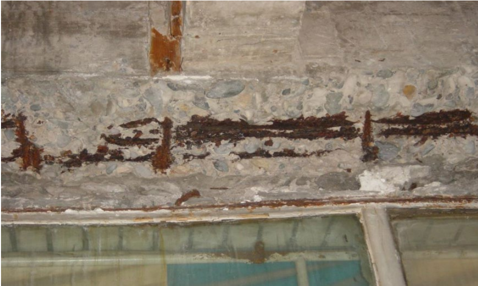
Figure 1.1 Rebar corrosion of RC slabs in a fine-art gallery of age 38 years by concrete carbonation. The building was constructed in 1962 with C25 concrete for the RC beams. The concrete binder is ordinary Portland cement (OPC), and the building was exposed to a rather dry environment with average temperature of 11 °C and average humidity of 57%. Source: courtesy of Tianshen Zhang.
