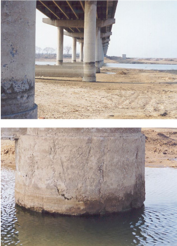
Figure 3.1 Concrete piers of a highway bridge across an inland river subject to frost action at the water level. The damage was present as the spalling of concrete cover and the coarse aggregates were exposed by spalling. The minimum temperature in winter reaches -10 to -15 °C in the region, the concrete grade was C30, and the service life of the bridge was 11 years at inspection. Source: courtesy of Xiaoxin Feng.
