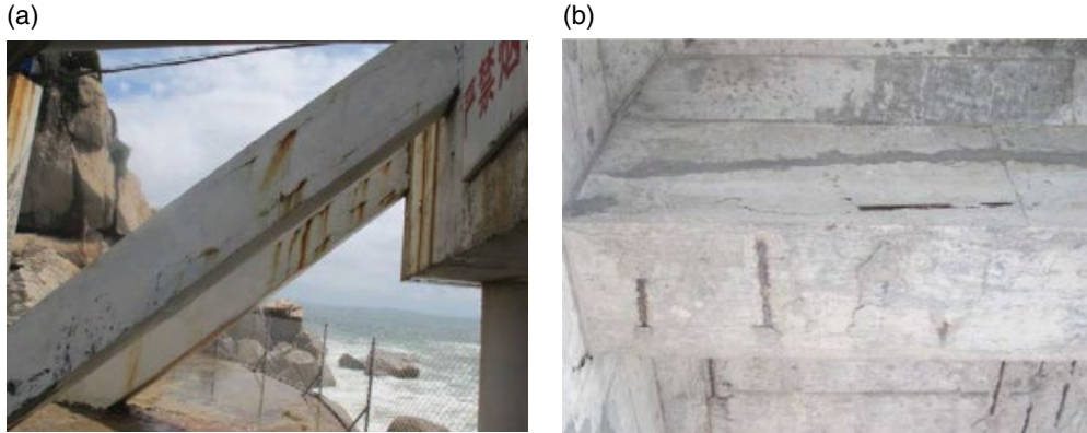
Figure 2.1 Corroded RC elements in a high-pile wharf on the southeastern coast of China. (a) Concrete cracking of 0.5 mm by chloride ingress on an inclined RC beam and (b) general spalling of concrete cover under an RC beam. The structure was put into service in 2001, the concrete grade was C30, and the design value of concrete cover was 50 mm. The in-situ strength of concrete was 35–48 MPa, and the concrete cover thickness inferior to design value was about 50% for these beams. Source: courtesy of Shengnian Wang.
