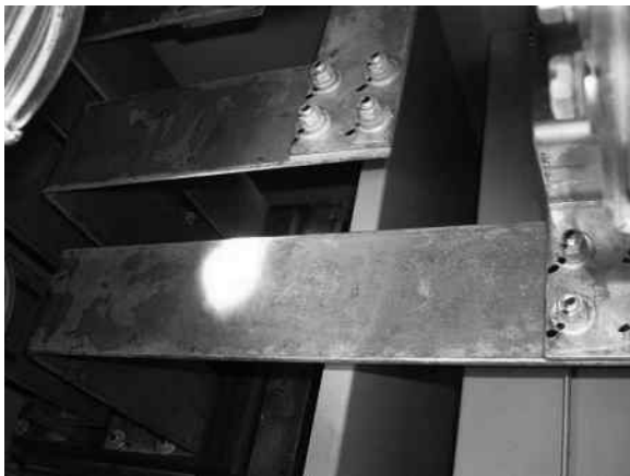
FIGURE 3.5 (See color insert.) Silver-flash plated copper bus after being shipped overseas. (Courtesy of Finishing.com, Online. Available: http://www.finishing.com/280/03.shtml ; the picture is taken by Steve Whatley.)
