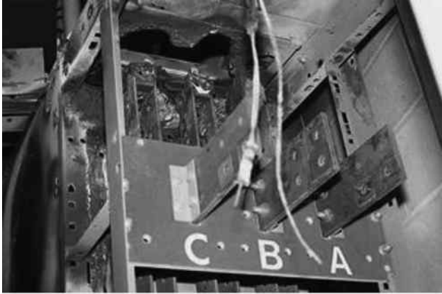
FIGURE 6.5 Failed LV switchboard. (From Ross B. Anatomy of a Meltdown , Electrical Construction and Maintenance, September 1, 2002, Online. Available: http://ecmweb.com/news/electric_anatomy_meltdown/ . With permission.)
