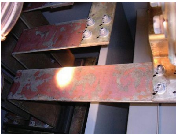
FIGURE 3.5 Silver-flash plated copper bus after being shipped overseas. (Courtesy of Finishing.com, Online. Available: http://www.finishing.com/280/03.shtml ; the picture is taken by Steve Whatley.)
