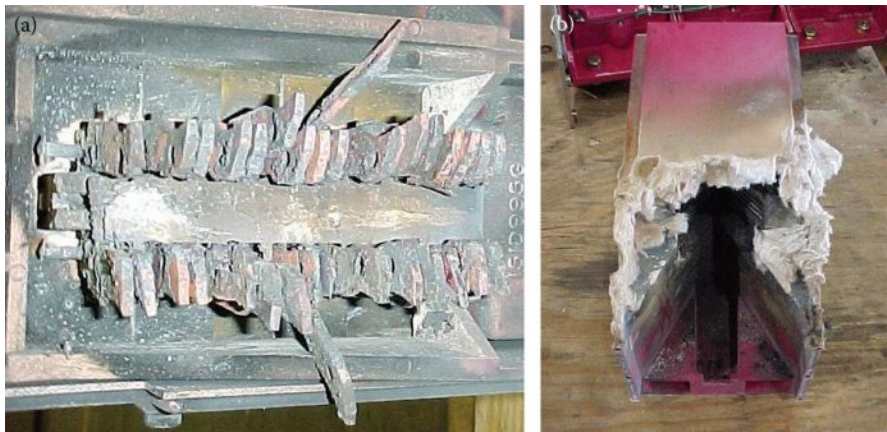
FIGURE 3.9 Images of the parts of the CB failed due to heavy corrosion and growth of silver whiskers: finger cluster (a) and arc chute (b).
