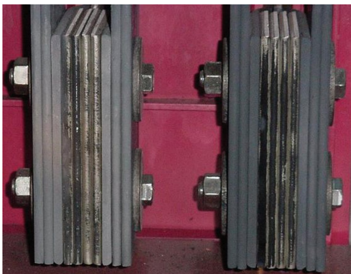
FIGURE 3.3 Heavy silver plating tarnish on copper bus after several months in service at an industrial facility.
