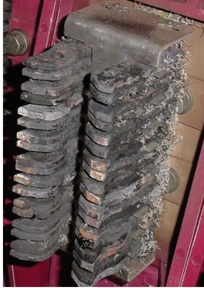
FIGURE 3.4 Finger cluster of corroded breaker after 2 months of service in a paper mill facility (pulp processing mill).
