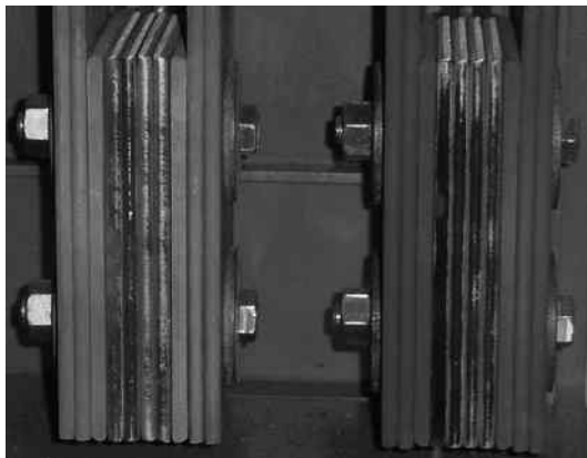
FIGURE 3.3 (See color insert.) Heavy silver plating tarnish on copper bus after several months in service at an industrial facility.
