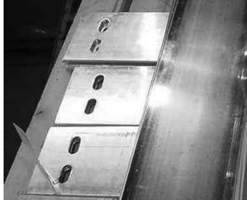
FIGURE 3.7 (See color insert.) Copper bus with silver flash stored for 12 months at a manufacturing facility with clean environment.
