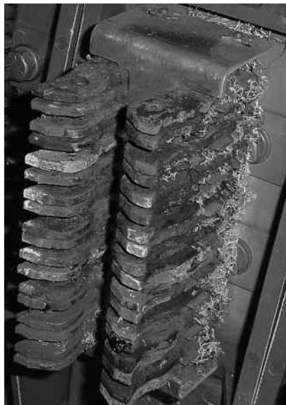
FIGURE 3.4 (See color insert.) Finger cluster of corroded breaker after 2 months of service in a paper mill facility (pulp processing mill).
