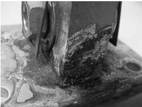
FIGURE 3.15 White rust on corroded galvanized steel parts of a CB exposed to moisture.
