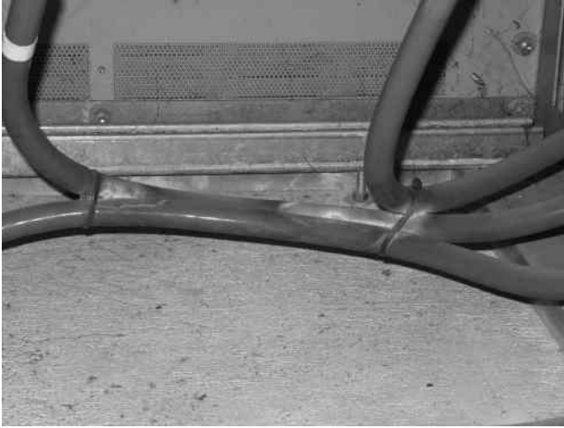
FIGURE 5.4 White powder/dust residue formed on 13 kV power cables that are tie-wrapped together, forming tight air spaces between each other. (From Brady J. Corona and Tracking Conditions in MC Switchgear Case Studies , Online. Available: http://www.irinfo.org/articles/article_8_1_2006_Brady.pdf . With permission.)
