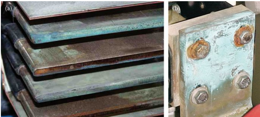
FIGURE 3.8 “Blue” and “green” corrosion of copper with silver flash on bus bars (a) and plate (b).
