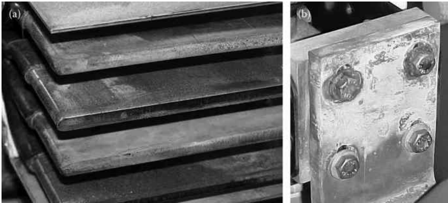
FIGURE 3.8 (See color insert.) “Blue” and “green” corrosion of copper with silver flash on bus bars (a) and plate (b).
