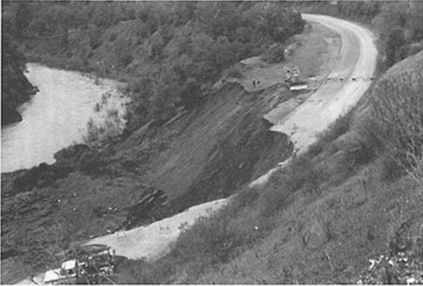
Figure 8.2 Slope failure at Sonoma County, California. (Reproduced by kind permission of California Division of Highways.)
