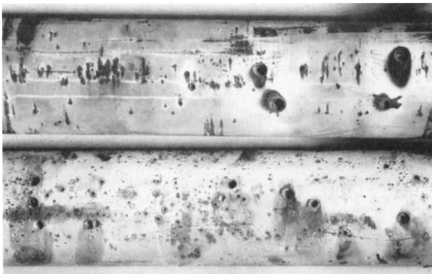
FIGURE 8.5.17 Blisters over pits on boiler tubes. (Courtesy of Babcock & Wilcox Co.)
