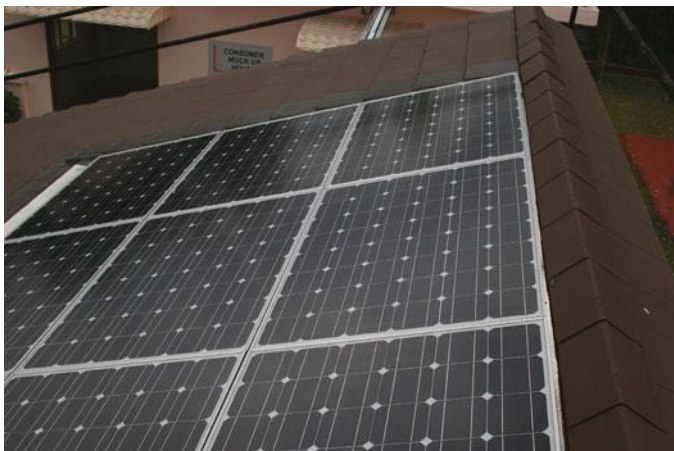
Figure 4.9 PV array composed of monocrystalline modules
