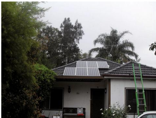
Figure 1.11 A residential PV system
