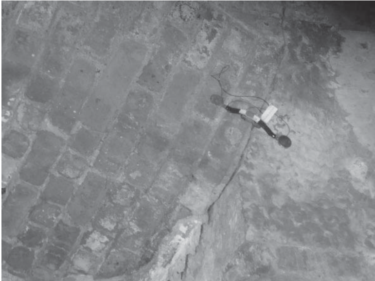
8.22 Crack sensor installed for monitoring a cracked masonry vault.
