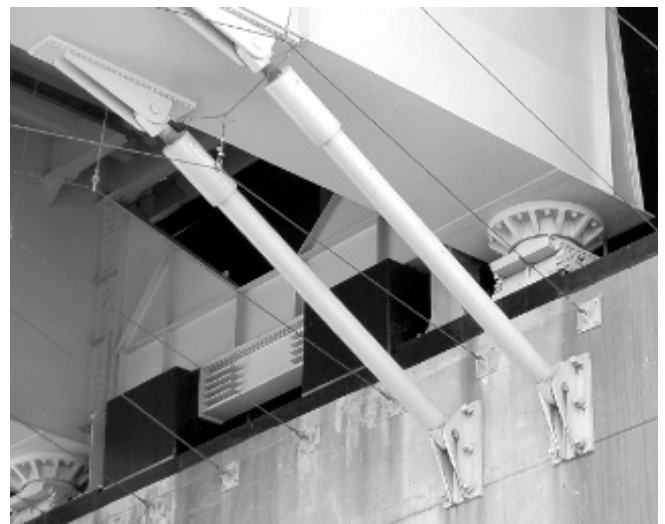
Figure 3.5: Vibration dampers are used under the Poplar Street bridge near the Riverfront in St. Louis. (Courtesy of Douglas P. Taylor of Taylor Devices, Inc.)
