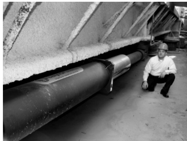
Figure 3.3: Large damper installed at the Los Angeles Regional Transportation Management Center. (Courtesy of Douglas P. Taylor of Taylor Devices, Inc.)
