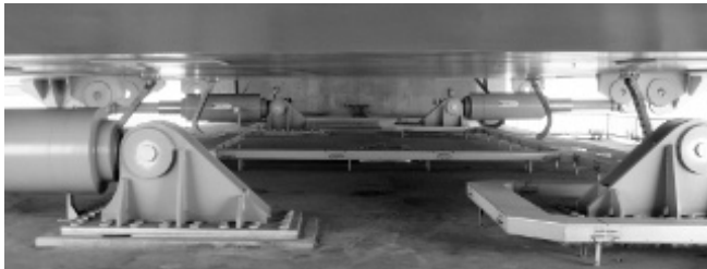
Figure 3.2: Spring-dampers installed under the Sutong Changjiang River Bridge in China. (Courtesy of Douglas P. Taylor of Taylor Devices, Inc.)
