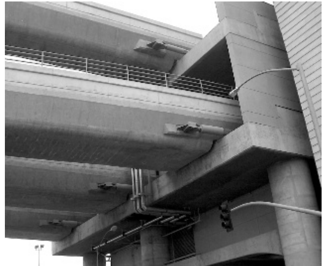
Figure 3.4: Dampers installed at the San Francisco International Airport. (Courtesy of Douglas P. Taylor of Taylor Devices, Inc.)
