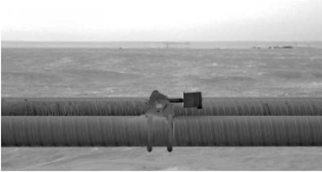
Figure 6.28: A Tuned Vibration Absorber (TVA) used on a pipeline in Alaska. The photograph shows a “hammer” type design in which a torsional spring in the base supports the arm and weight. The length of the arm and number of weights is variable. The photograph was taken at a BP-operated facility in the Prudhoe Bay area of Alaska, north of the Arctic circle, where the Trans-Alaska pipeline begins. (Courtesy of Evan D. Kane, February 2009)
