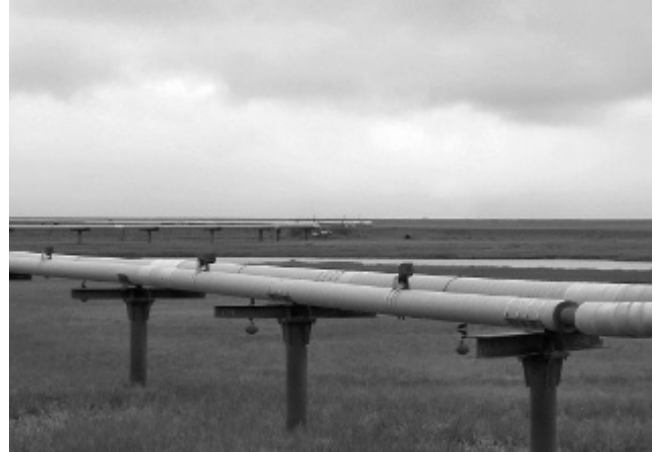
Figure 6.29: Two designs of Tuned Vibration Absorbers (TVAs) used on pipelines in Alaska. The photograph shows (1) a hanging spring-mass design (classic vibration absorber) and (2) a “hammer” type design in which a torsional spring in the base supports an arm and weight. The absorbers are tuned to absorb three main frequencies. They are used for most of the pipeline, starting at an anchored support in the middle and alternating through the three frequencies on spans between sliding supports until the line reaches an expansion loop. The photograph was taken at a BP-operated facility in the Prudhoe Bay area of Alaska, north of the Arctic circle, where the Trans-Alaska pipeline begins. (Courtesy of Evan D. Kane, February 2009)
