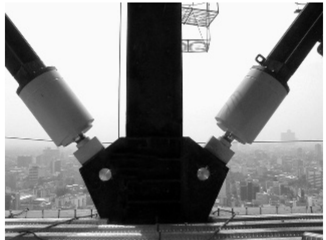
Figure 9.30: Mega-brace dampers for Torre Mayor building. (Courtesy of Douglas P. Taylor of Taylor Devices, Inc.)
